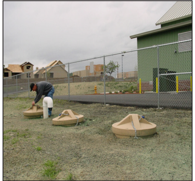
Dave McFall, manager for Eagle Point School District’s construction projects inspects one of the underground water storage tanks that pre-cools water.
