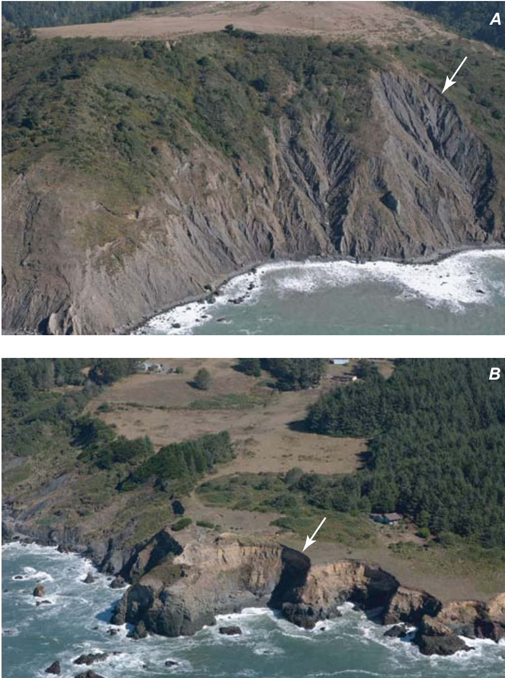
Figure 14. Areas of the highest cliff retreat rates in the Eureka region. The white arrows point to the feature interpreted as the cliff edge: A) loose, unconsolidated material in landslide complex is eroding rapidly via the formation of rills and gullies in the vicinity of False Cape, ~7 km north of Cape Mendocino (see Figure 10A). The cliff at this site retreated over 150 m in a 70-year time period; and B) rapid erosion of unlithified marine terrace deposits that overlie stronger bedrock material resulted in erosion rates > 2 m/yr near Elk Cape (see Figure 10A). (Photos copyright (c) 2002-2007 Kenneth & Gabrielle Adelman, California Coastal Records Project, www.californiacoastline.org ).
