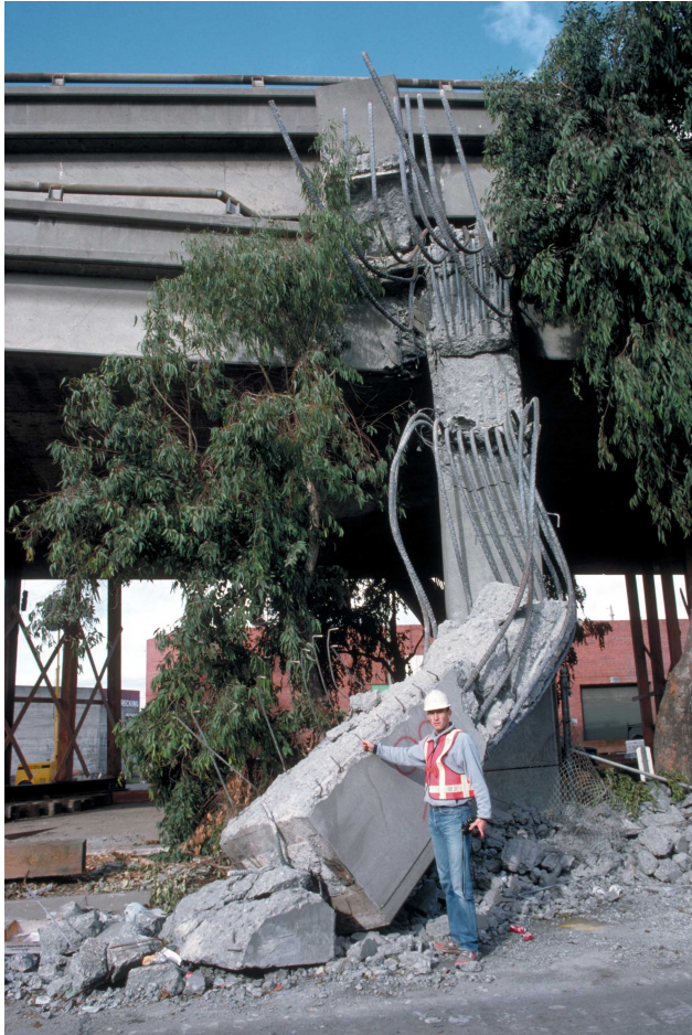
23. Support-column failure and collapsed upper deck, Cypress viaduct. [H.G. Wilshire, U.S. Geological Survey]
