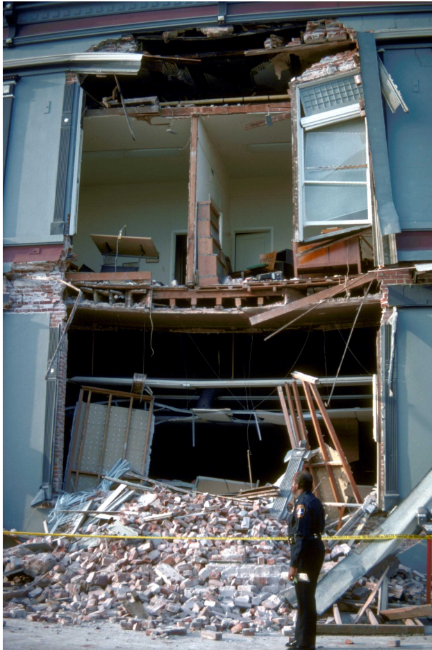
81. Close-up of collapsed wall of unreinforced masonry, Medico Dental Building in the Pacific Garden Mall. [H.G. Wilshire, U.S. Geological Survey]
