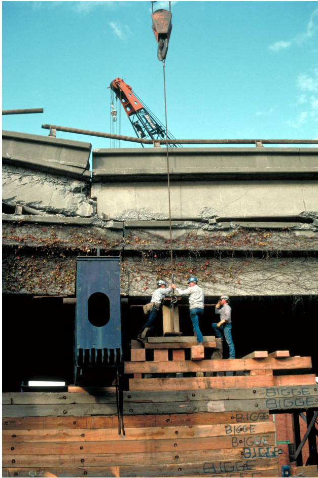
28. Temporary support structures emplaced to prevent further collapse, Cypress viaduct. [H.G. Wilshire, U.S. Geological Survey]
