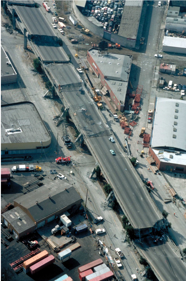
18. Aerial view of collapsed sections of the Cypress viaduct of Interstate Highway 880. [H.G. Wilshire, U.S. Geological Survey]
