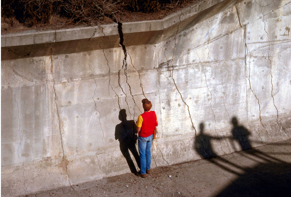
59. Prominent N. 15 o W.-trending extensional cracks up to 12 cm (4.7 in.) wide in concrete spillway to Austrian Dam, north abutment. [G.R. Fisher, U.S. Geological Survey]
