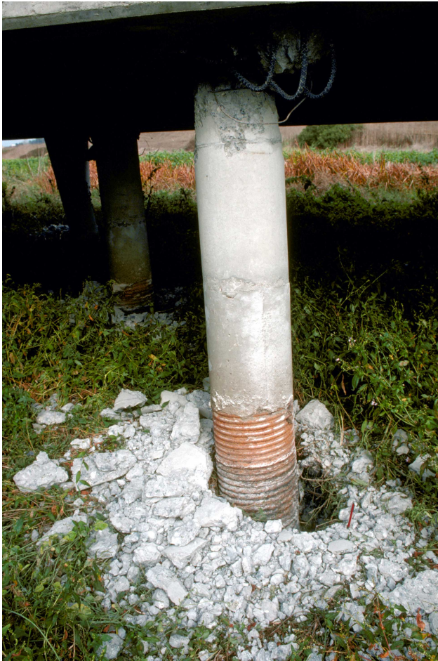
98. Support column of bridge across Struve Slough, Highway 1. Enlargement of hole where support enters the ground is an effect of lateral shaking, which caused the concrete to break up where the column joined the bridge and was instrumental in the roadbed collapse. [H.G. Wilshire, U.S. Geological Survey]
