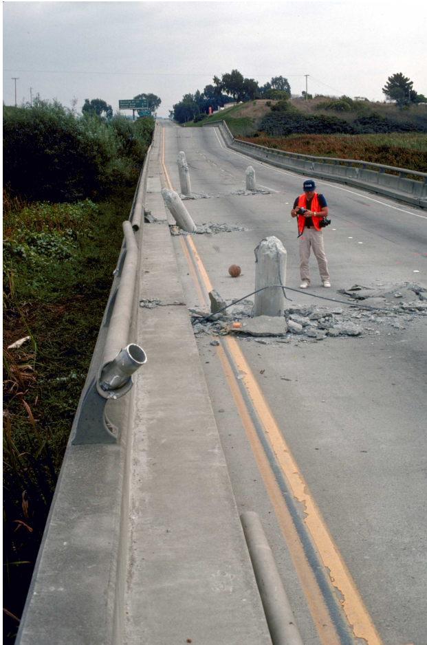
97. Support columns of Highway 1 bridge across Struve Slough protrude through roadbed. This resulted from collapse of the roadbed after the effects of lateral shaking shown in photo 98. [H.G. Wilshire, U.S. Geological Survey]
