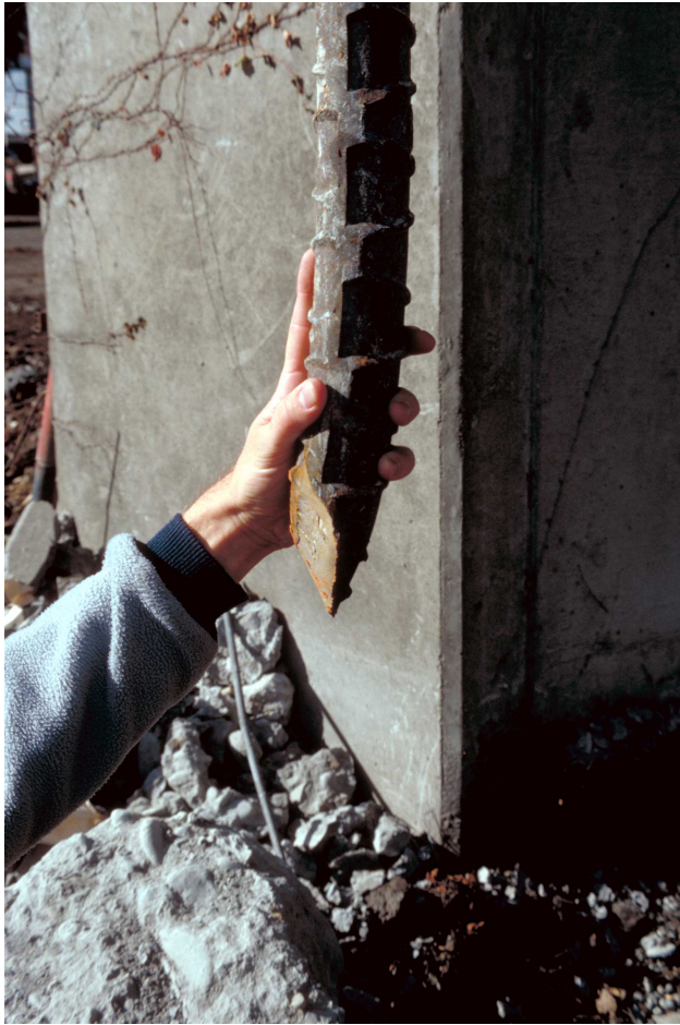
27. Sheared reinforcement bar, Cypress viaduct. [H.G. Wilshire, U.S. Geological Survey]
