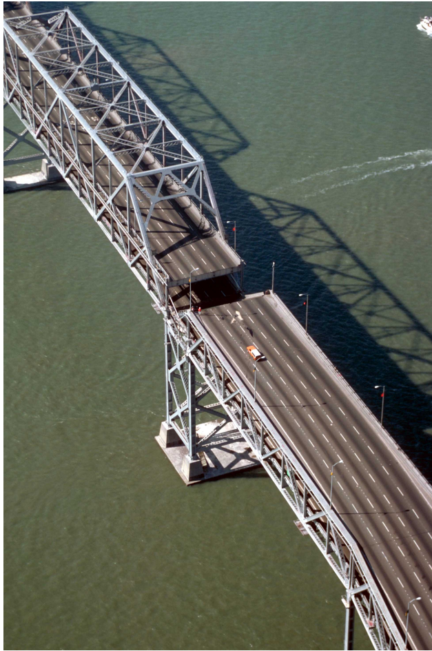
16. Aerial view of the collapsed section of the San Francisco-Oakland Bay Bridge. View westward. [C.E. Meyer, U.S. Geological Survey]
