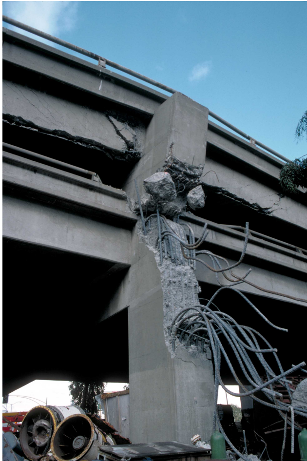
24. Bent reinforcement bars in failed support column, Cypress viaduct. [H.G. Wilshire, U.S. Geological Survey]
