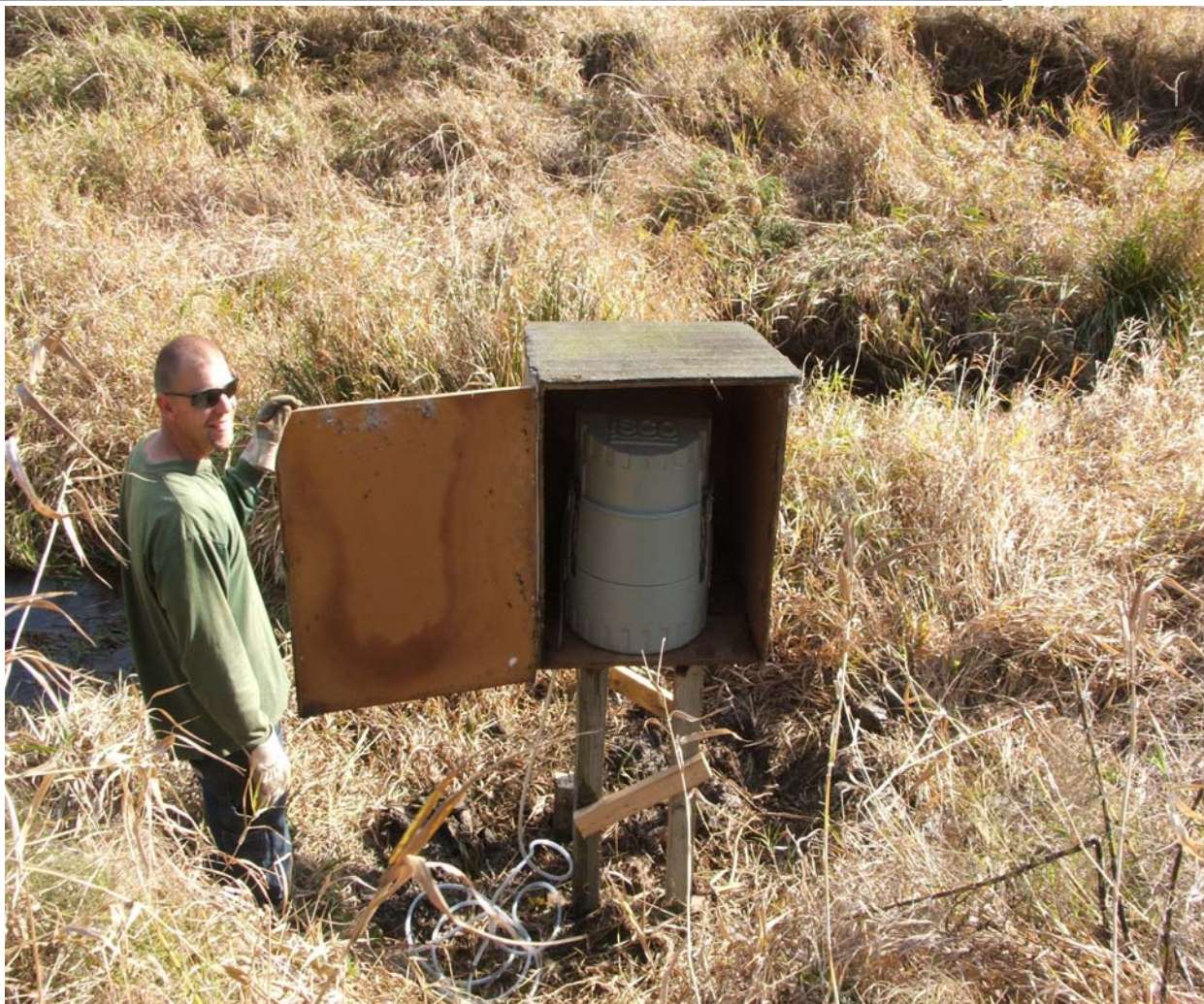
Photo 11. Blacks Creek VEMCO monitoring station.
