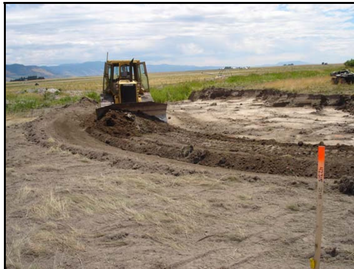
D5 Dozer grading material from floodplain in preparation for bankfull channel excavation by track-hoe. July 2006
