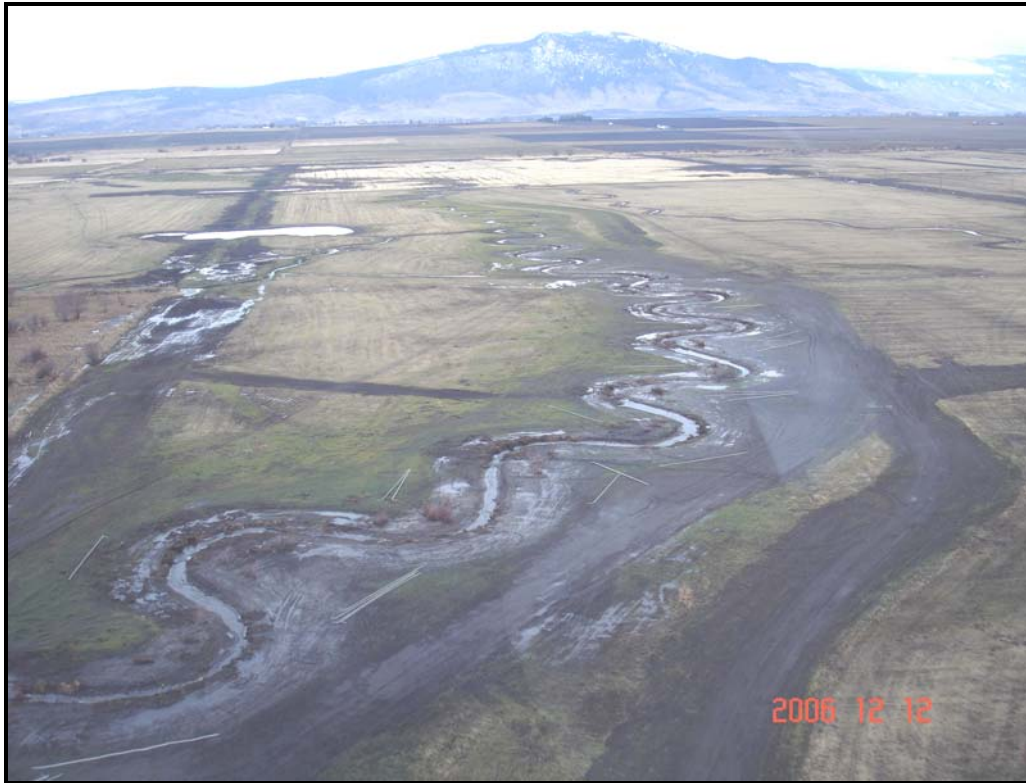
Upstream reach of End Creek (Rice) Restoration Channel, viewing east (downstream) towards South Fork Willow Creek confluence. Note reclaimed channelized reach in left corner of photo and floodplain ponds incorporated into reclamation plan. December 2006
