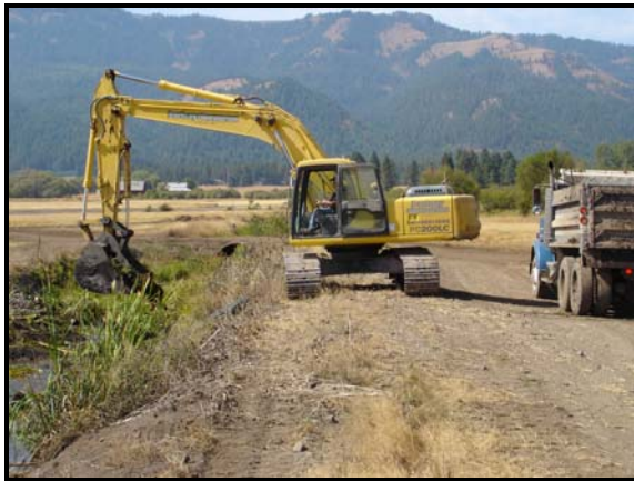
Excavator prepares excavate and load sedge matt from the channelized End Creek alignment prior to reclamation (backfilling). September 2006.
