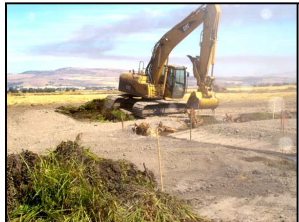
Excavator installing sedge/rush mats along outside stream meander on rootwad revetment. September 2006
