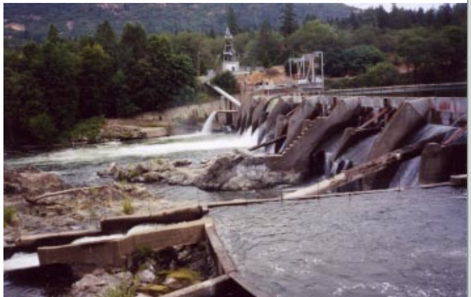
Removal of Savage Rapids Dam would improve fish passage to over 500 miles of upstream habitat.
