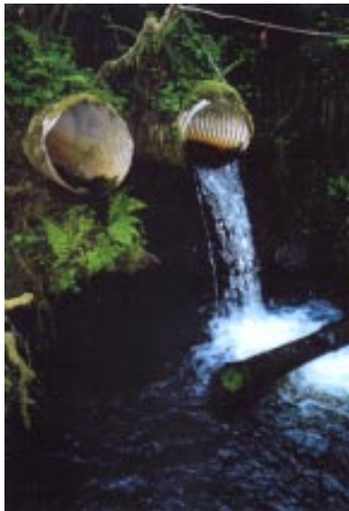
Fish passage was blocked on Boxler Creek by two culverts.
