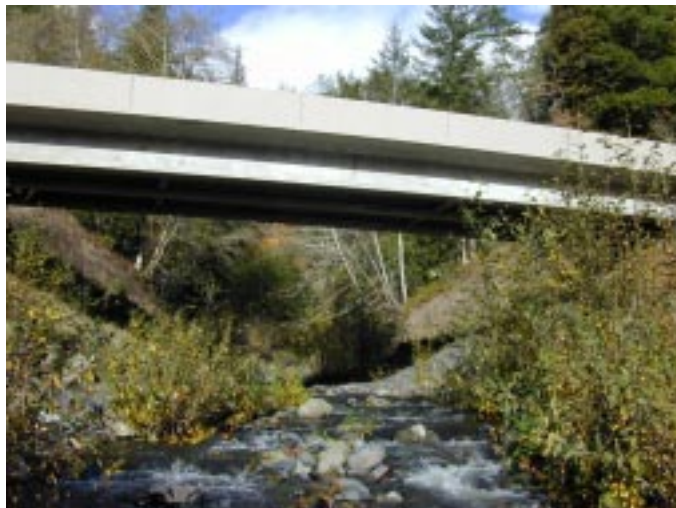
Deep Creek restored to its natural flow after installation of a bridge.
