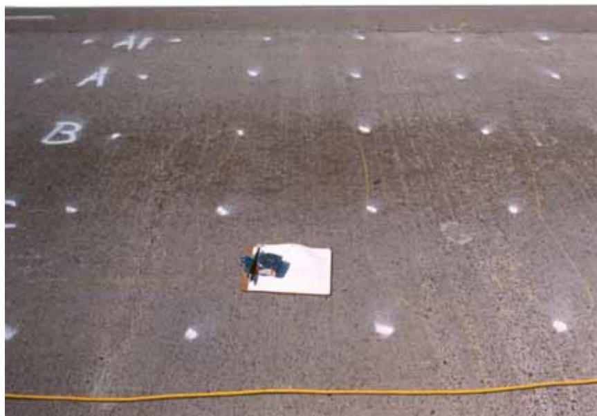
Figure 25. Photograph showing typical cracking found in the northbound deck of the U.S. 41 test section LMC.
