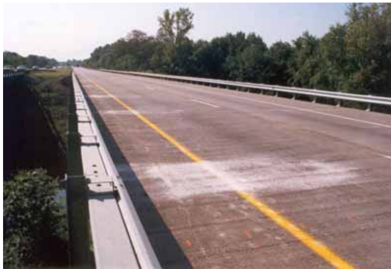
Figure 9. Photograph showing the eastbound deck of U.S. 52 over Raymond Run in Columbus, OH. The overlay is latex-modified.
