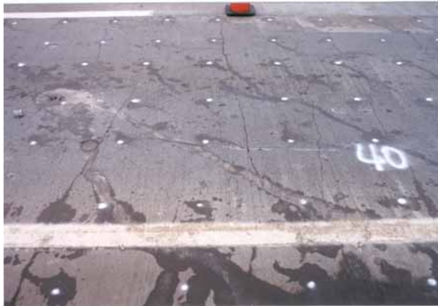
Figure 26. Photograph showing typical cracking associated with the southbound test section of U.S. 41 SFC.
