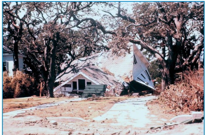
Damage from Hurricane Camille, August 17, 1969/NOAA
