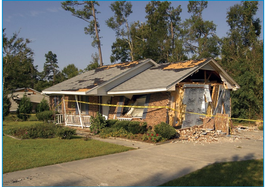
Hurricane Frances tornado damage, Sumter County, SC September 6, 2004/ Photo by Marvin Nauman/FEMA
