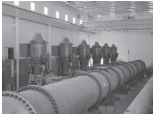
Construction is continuing on the San Juan-Chama Drinking Water Project's Raw Water Pump Station. The station is located just south of the Alameda Open Space Area off Alameda Boulevard NE.
