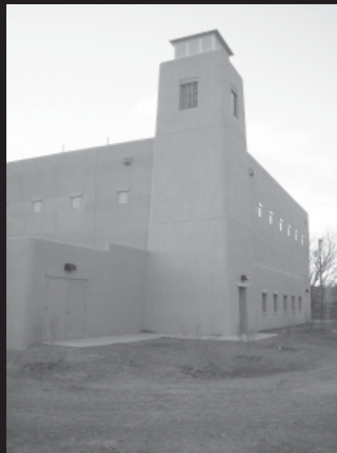
Construction is nearing completion on the Raw Water Pump Station. Based on input from residents in the area, the pump station was designed to resemble an old Mission-style church to better blend in with its surroundings.
