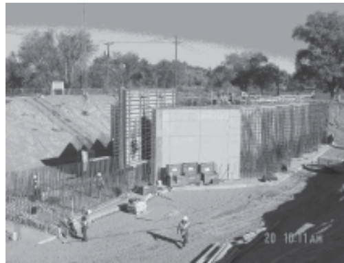
Crews Continuing Work on the Raw Water Pump Station in Northwest Albuquerque
