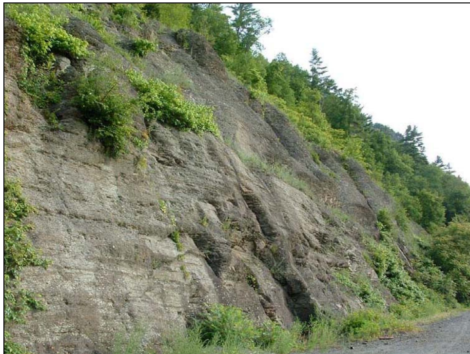
Figure 119. Shale Scree Slope in Delaware Water Gap National Recreation Area (along Route 209, near Milford, in Pennsylvania). June 2006.
