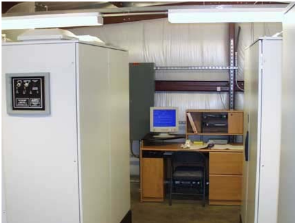
Dispersal Barrier Control Room (Photo courtesy of Phil Moy, Wisconsin Sea Grant)
