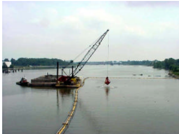
Saginaw River, Michigan Sediment Cleanup Using Sealed Dredge Bucket and Silt Curtain to Prevent Spread of Contamination (Photo courtesy of U.S. Fish and Wildlife Service)
