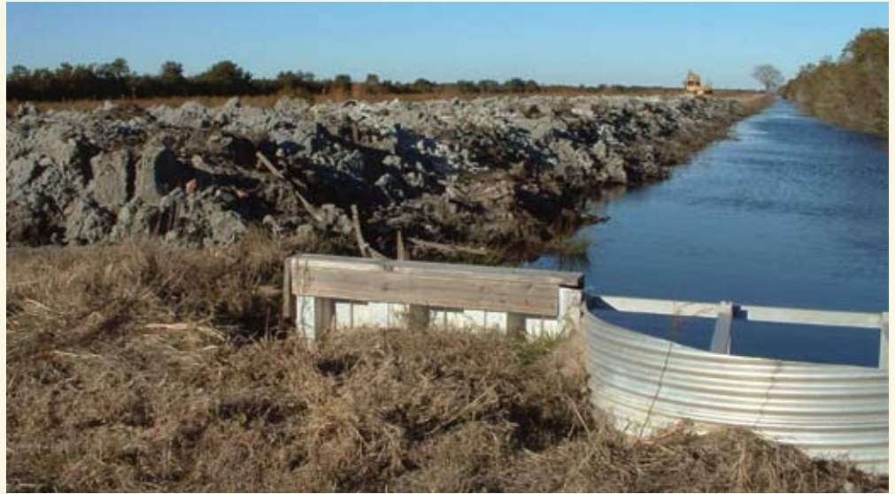
Raised roads act as levees to re-flood historically drained peatlands at Pocosin Lakes National Wildlife Refuge in North Carolina. (Sara Ward/USFWS)
