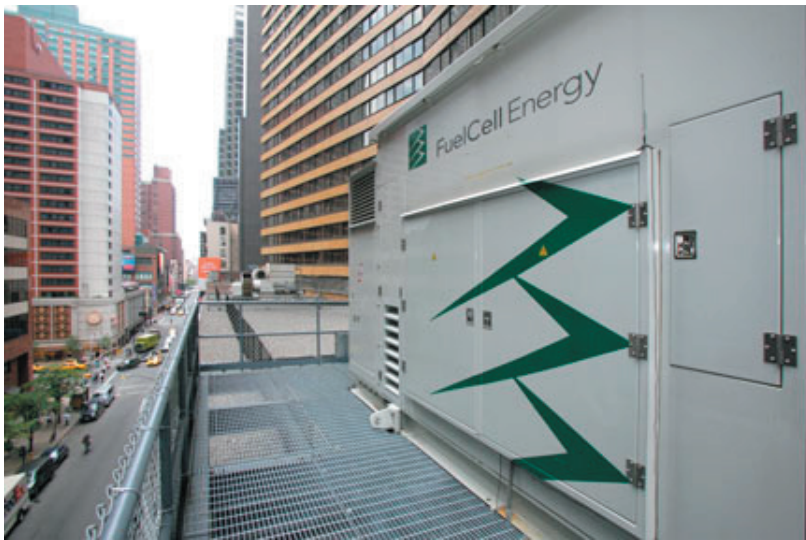
A 250-kilowatt fuel cell, part of the system that generates electricity and heats water for a Sheraton hotel in New York.
