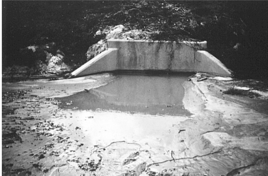
Figure VI-15--Sediment Deposition in Culvert
