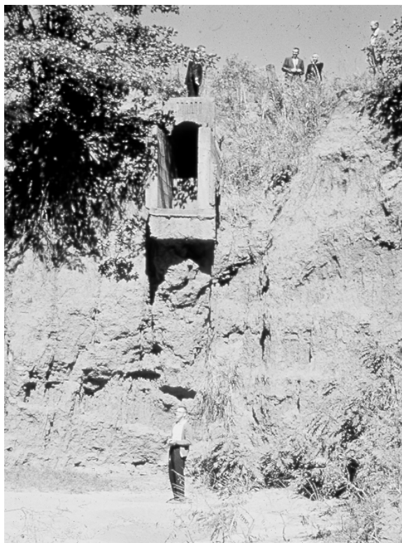
Figure VI-13--Stream Degradation at Culvert Outlet
