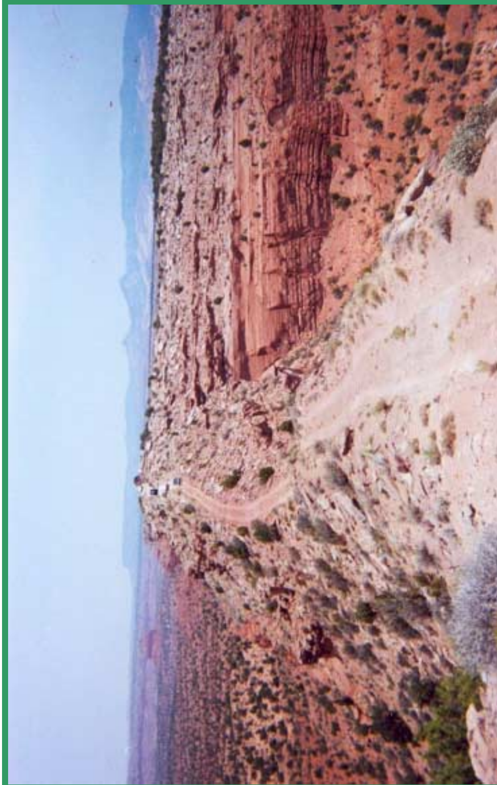
Natural Bridge provided a narrow access road to Sweetwater-2 AML Reclamation Project. Note trucks in the background for scale.
