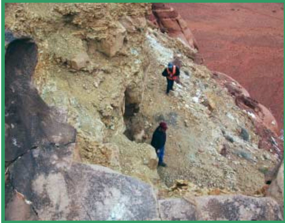
Monument Valley-4 Project, Rock Door Mine: Poly Urathane Foam Portal Closure. This Portal is several hundred feet high. Monument Valley is directly east of this vertical rock face. Workers were tied to safety ropes, for safety, while completing this closure.
