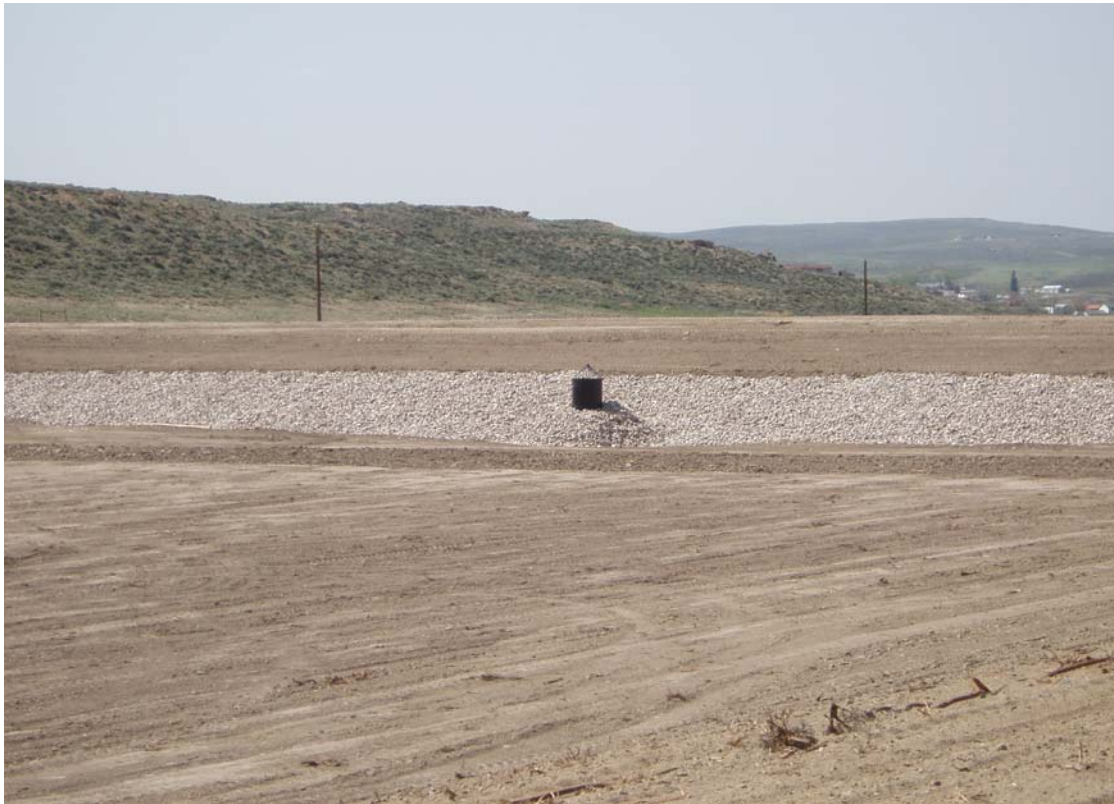
Photo 3. Hanna #4 mine – Phase 2 run-off attenuation and mass excavation project includes this detention structure and armoring of the stream channel to protect the town of Hanna, WY.
