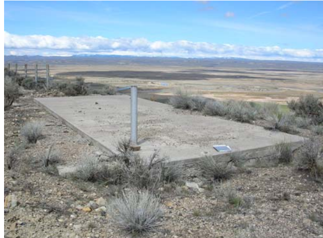
Photo 5. Cast-in-place concrete slab closure on vertical opening 2 in the Brazier Demonstration project. April 24, 2007.
