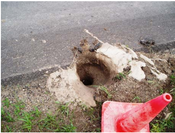
Williams County Road 9 Phase I Project completed pressurized grout injection hole along county road
