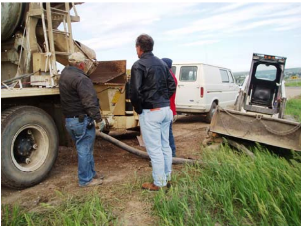
Williams County Road 9 Phase II Project pressurized grout injection along county road
