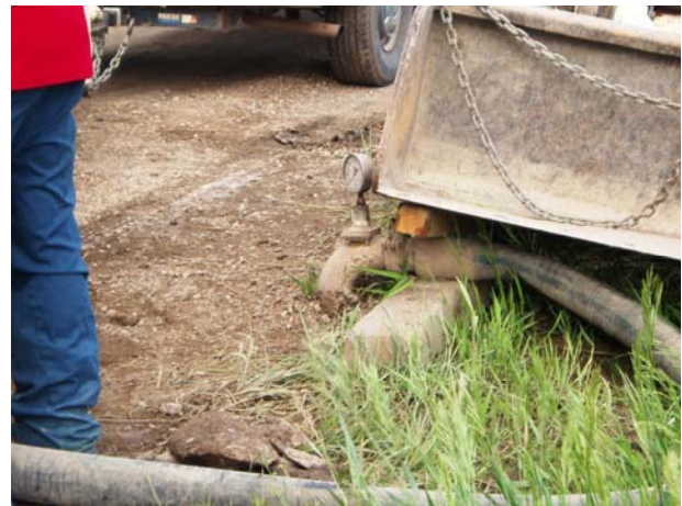
Williams County Road 9 Phase II Project injection of pressurized grout into drilled injection hole
