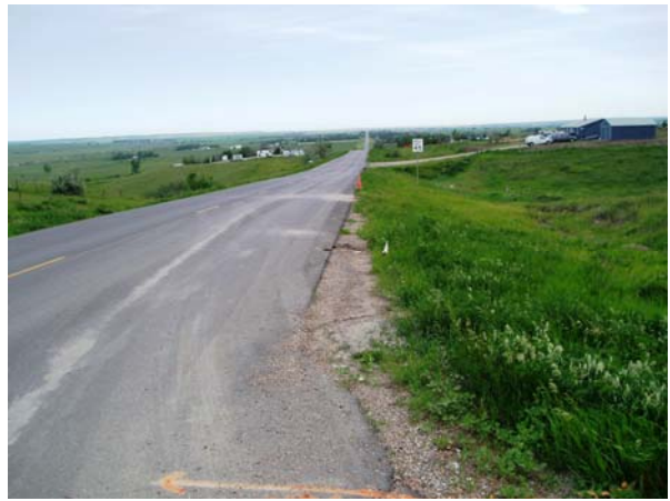
Williams County Road 9 Phase I Project pressurized grout injection along county road
