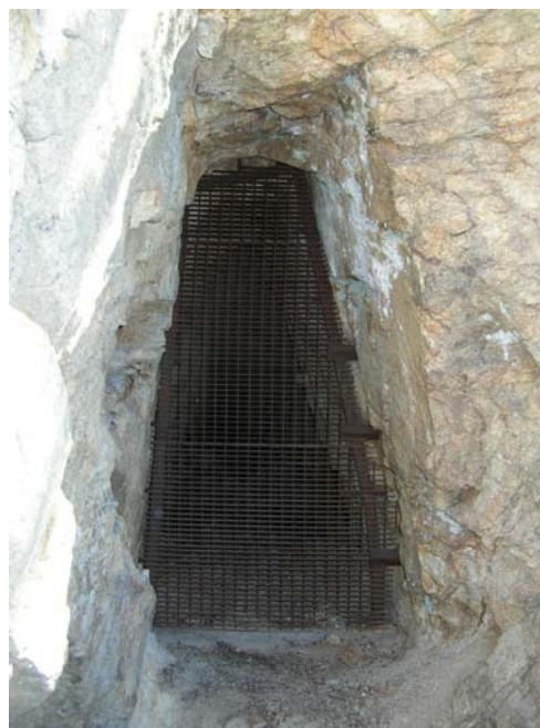
Photo 1. Steel grate closure in portal SG-6 of the Good Hope project. August 8, 2006.
