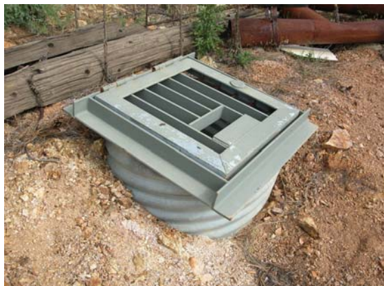
Photo 2. Corrugated metal pipe with locking access door closure in vertical opening S-33 of the Golden Harp project. August 9, 2006.
