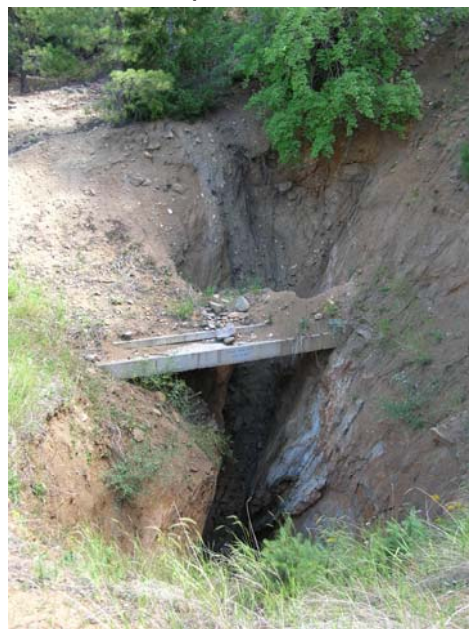
Photo 3. Damaged pre-cast concrete panel closure of vertical opening S-47 of the Golden Harp project. August 9, 2006.
