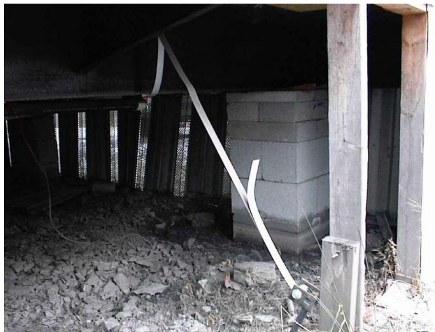
Figure 2 Hurricane straps required by building code in states in which trailer were selected for the study in Ohio, Tennessee, Alabama, and Indiana
