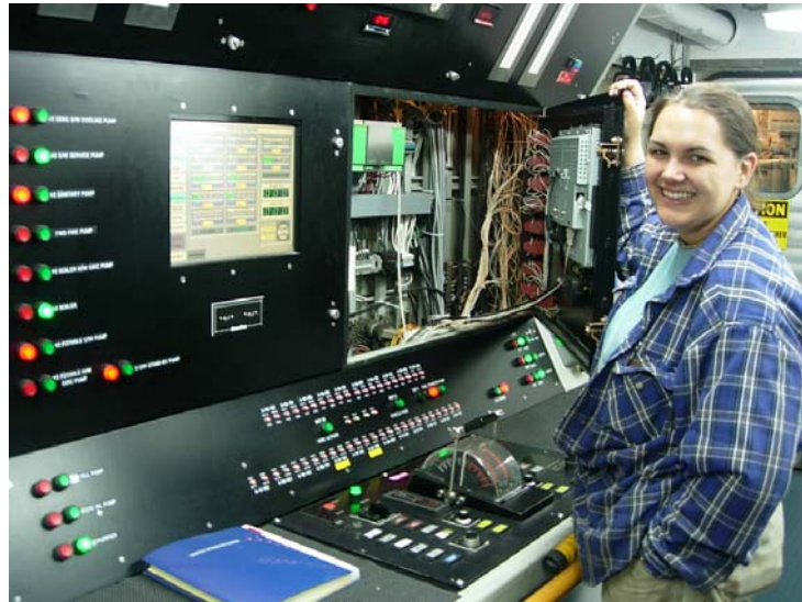
Third Assistant Engineer Kelly Baughman at the center console in the engine room onboard the RAINIER. Kelly fired up the engines to get the ship underway this morning!
