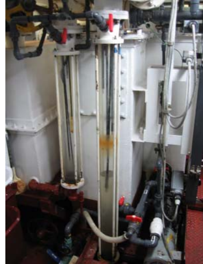
The Marine sanitation Device (MSD) which treats the sewage produced aboard the NOAA ship RAINIER
