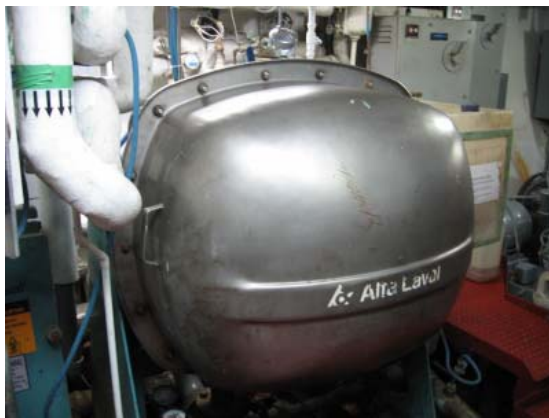
One of the two evaporators on the NOAA ship RAINIER which processes salt water into fresh water
