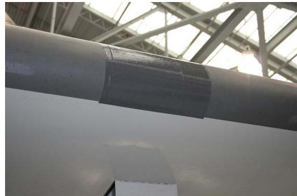
The small, smooth patch on the wing where the repair had been made
