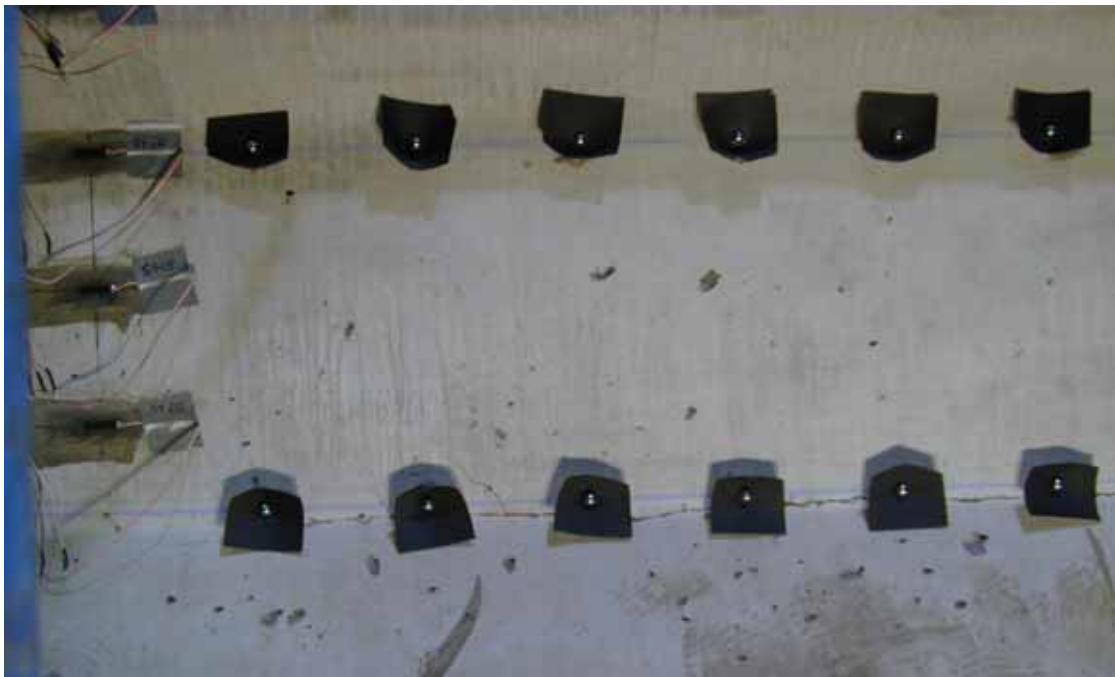
Figure 28. Photo. Crack at south base of Girder 28S web at a load of 2,000 kN (450 kips).
