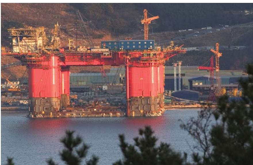
Atlantis floating production platform under construction in Korea. Photo and artist rendition courtesy of BP Exploration & Production.
