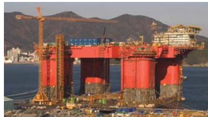
Atlantis floating production platform under construction in Korea. Photo courtesy of BP Exploration & Production.
