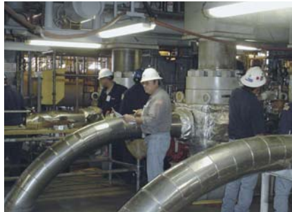
MMS inspectors examine the incoming flowline risers of the Thunder Horse semisubmersible production platform.
