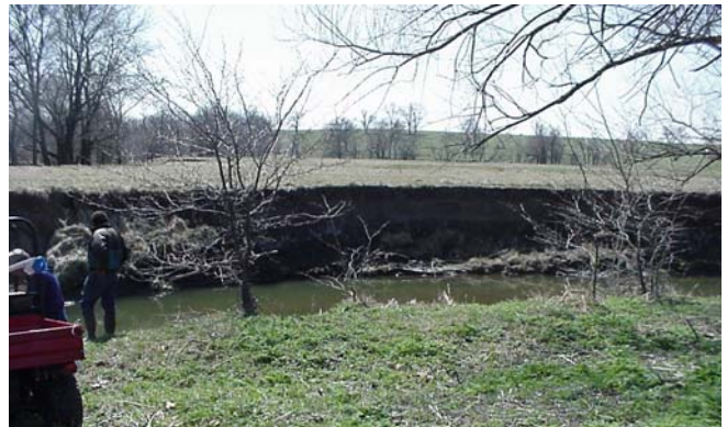
These are before and after photos of a streambank stabilization project. The photo above shows major erosion along the bank resulting in loss of valuable farmland.
