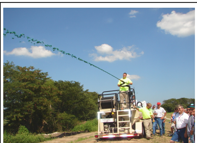
A hydro seeder can quickly establish cover to a newly developed site to reduce soil erosion and improve water quality.
