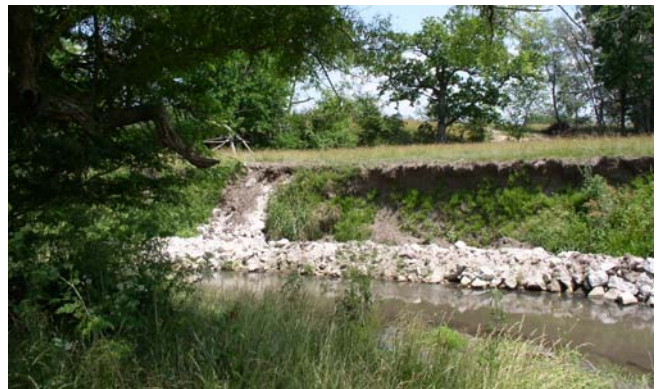
The photo below shows the same site after stone toe protection and stream barbs where placed in designated locations to control the amount of sediment entering Illinois' lakes, streams and backwater areas.
