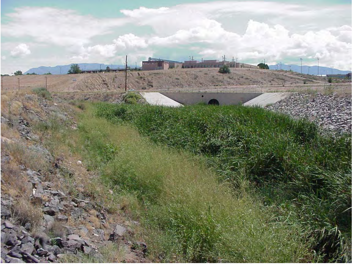
South Diversion Channel at Motel 6 on Avenida de Cesar Chavez (Upper South Diversion)
