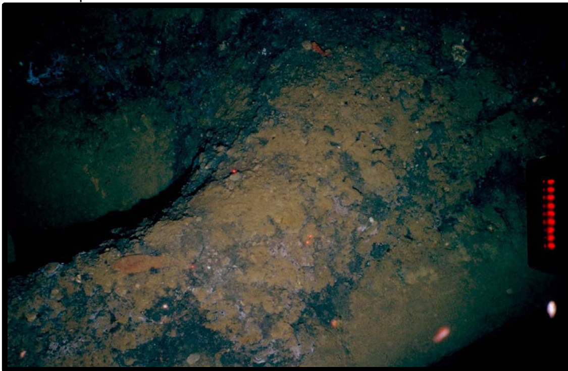
Photo 10 - Accumulations of suspected muds and cuttings on top of substructures at the base of the Garden Banks Area Block 128 platform structure.
