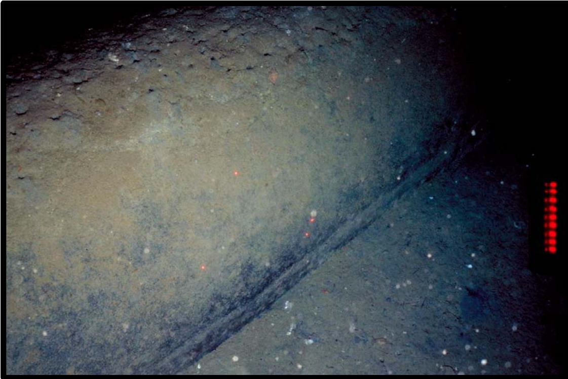
Photo 25 - Accumulations of suspected discharge along the northeast Viosca Knoll Area Block 780 platform. Depths of the observed accumulations ranged from approximately a few inches to a slight dusting.
