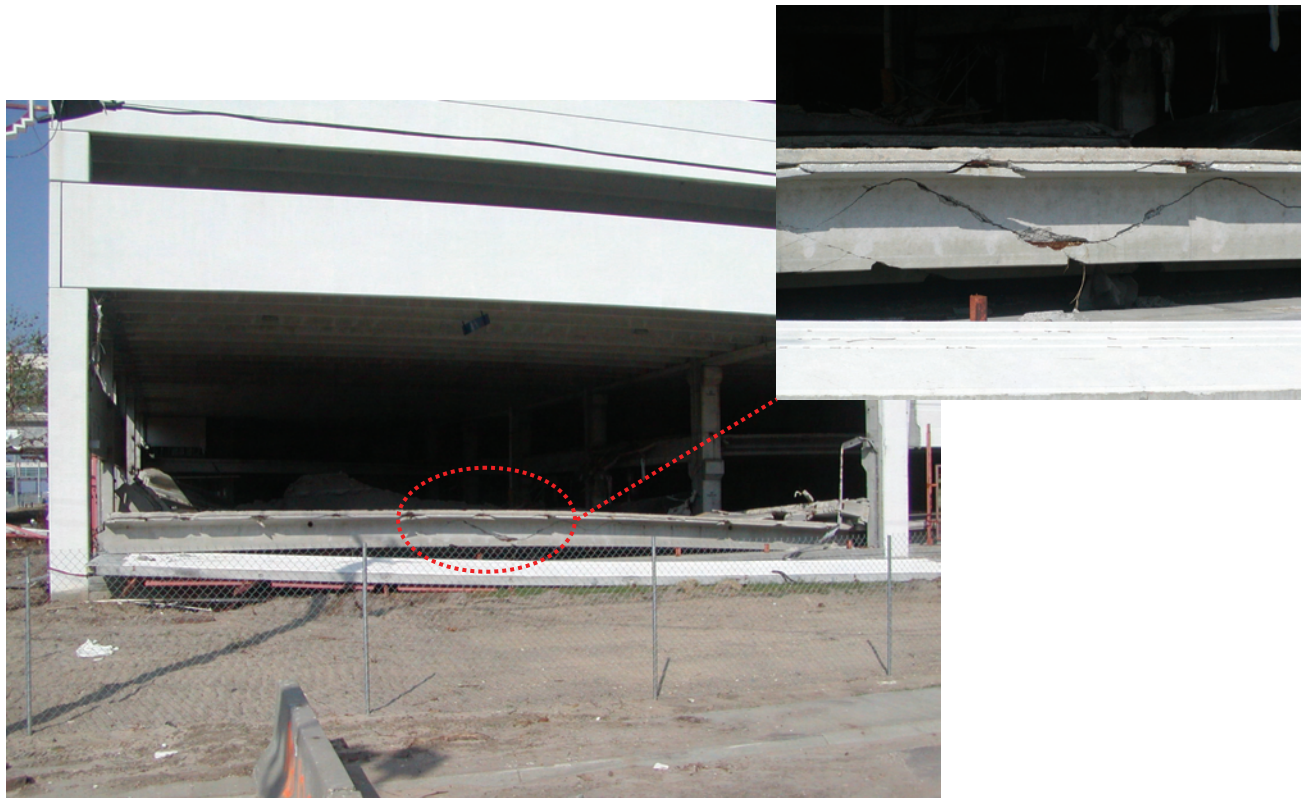
Figure 2-27 Negative bending failure of a prestressed double-tee floor system due to uplift forces (Hurricane Katrina, 2005).
