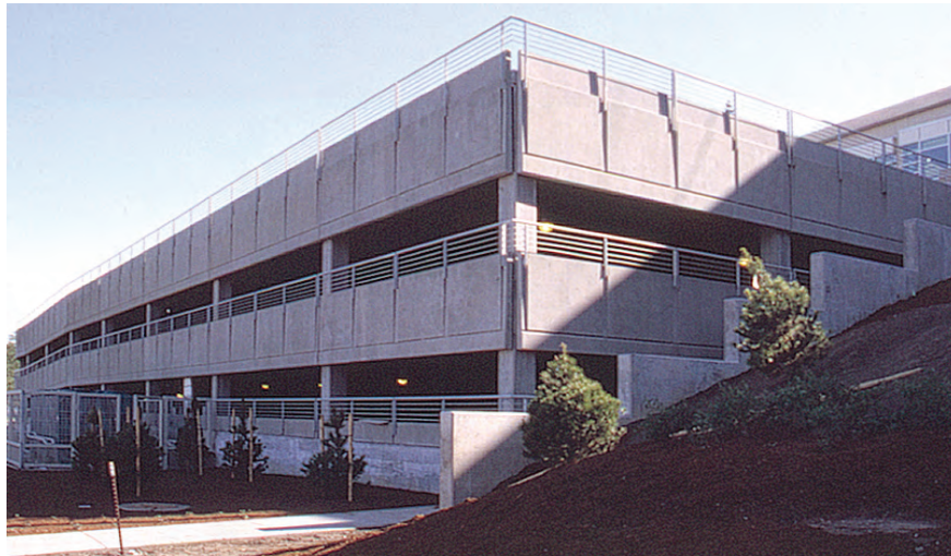
Figure 4-2 Parking garage. Open structural systems allow water to pass through with minimal resistance, and interior ramps allow for easy ingress and vertical circulation.
