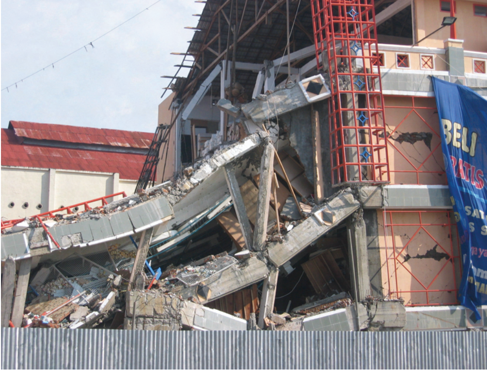
(a) Beam-column connection failures
