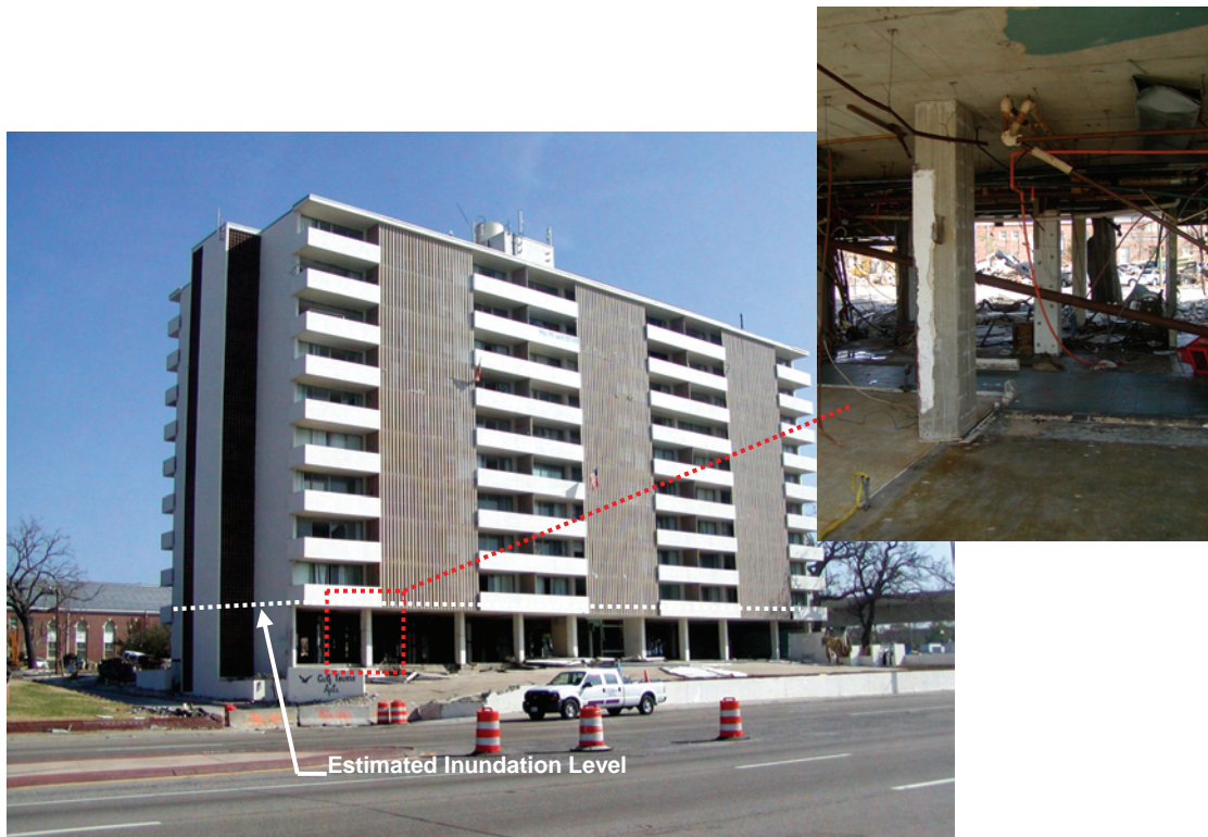
Figure 2-22 Gulf Tower Apartment building suffered substantial non-structural damage at the ground floor level, but remained structurally sound (Hurricane Katrina, 2005).
