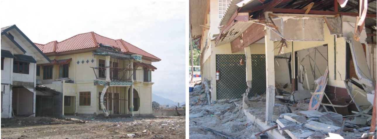
Figure 2-17 Damage to non-engineered concrete columns due to debris impact (Photos courtesy of M. Saatcioglu, A. Ghobarah and I. Nistor, CAEE, 2005).
