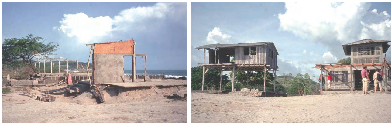
Figure 2-11 Beach houses with varying levels of damage in El Popoyo, Nicaragua (1992 Nicaragua Tsunami). All three houses are in the same vicinity.
