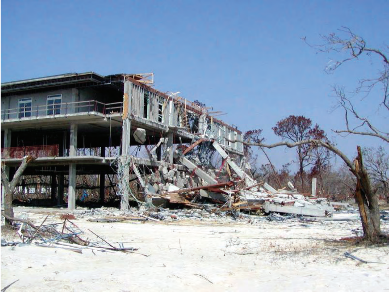
Figure 2-28 Concrete frame of three-story apartment building that partially collapsed due to failure of the post-tensioned flat slab in the bay closest to the Gulf of Mexico (Hurricane Katrina, 2005).
