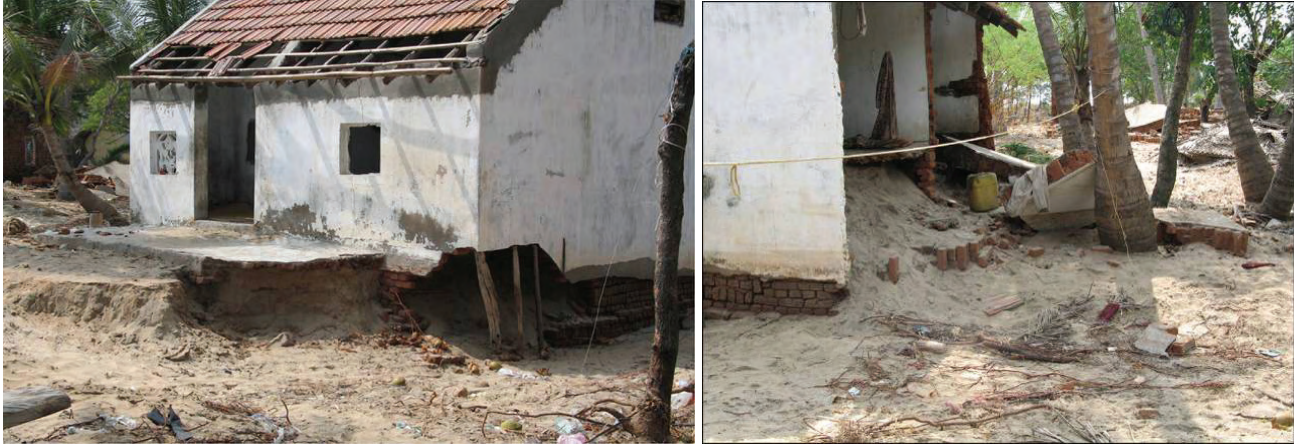
Figure 2-14 Damaged masonry beach house in Devanaanpattinam, India (2004 Indian Ocean Tsunami).
