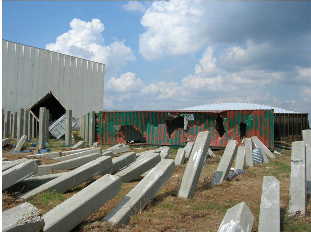
Figure 2-26 Failure of prestressed piles due to damming effect of shipping container (Hurricane Katrina, 2005).
