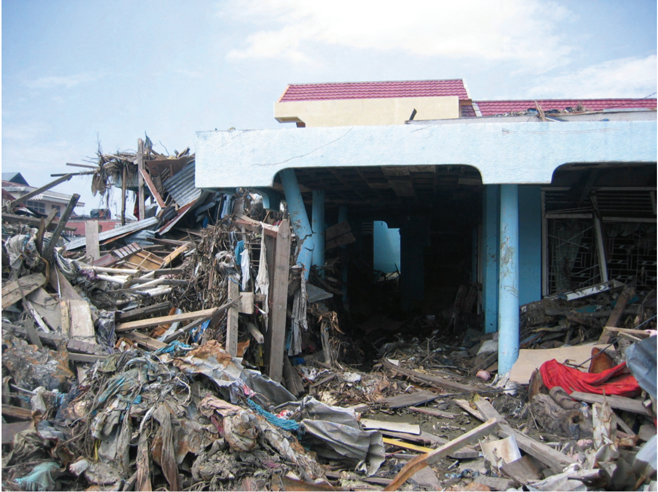
Figure 2-18 Damage to corner column due to debris damming (Photo courtesy of M. Saatcioglu, A. Ghobarah and I. Nistor, CAEE, 2005).
