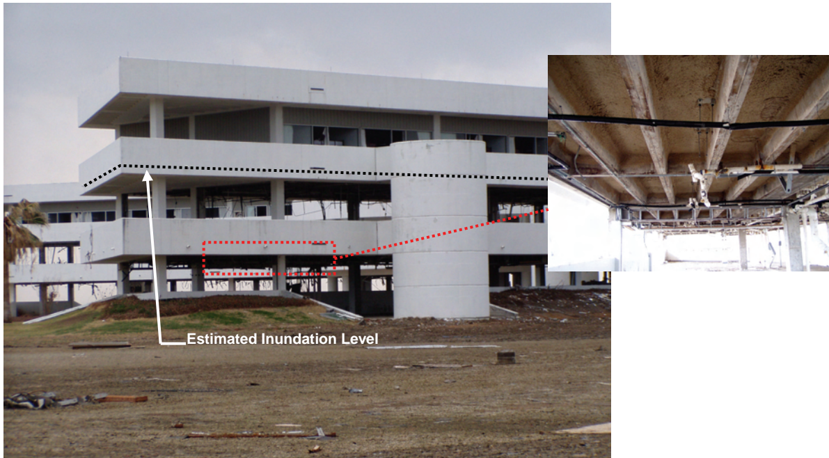
Figure 2-23 Pass Christian office building with cast-in-place concrete pan joist floor system that suffered non-structural damage at first two floors but no structural damage (Hurricane Katrina, 2005).
