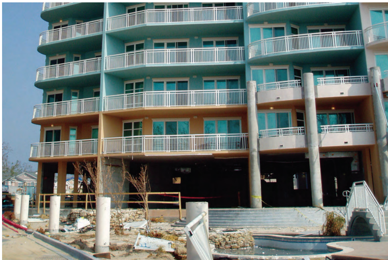
Figure 2-24 Condominium building in Gulfport, Mississippi, with wave and storm surge damage to non-structural elements at the ground floor, but no reported structural damage (FEMA 549, 2006).
