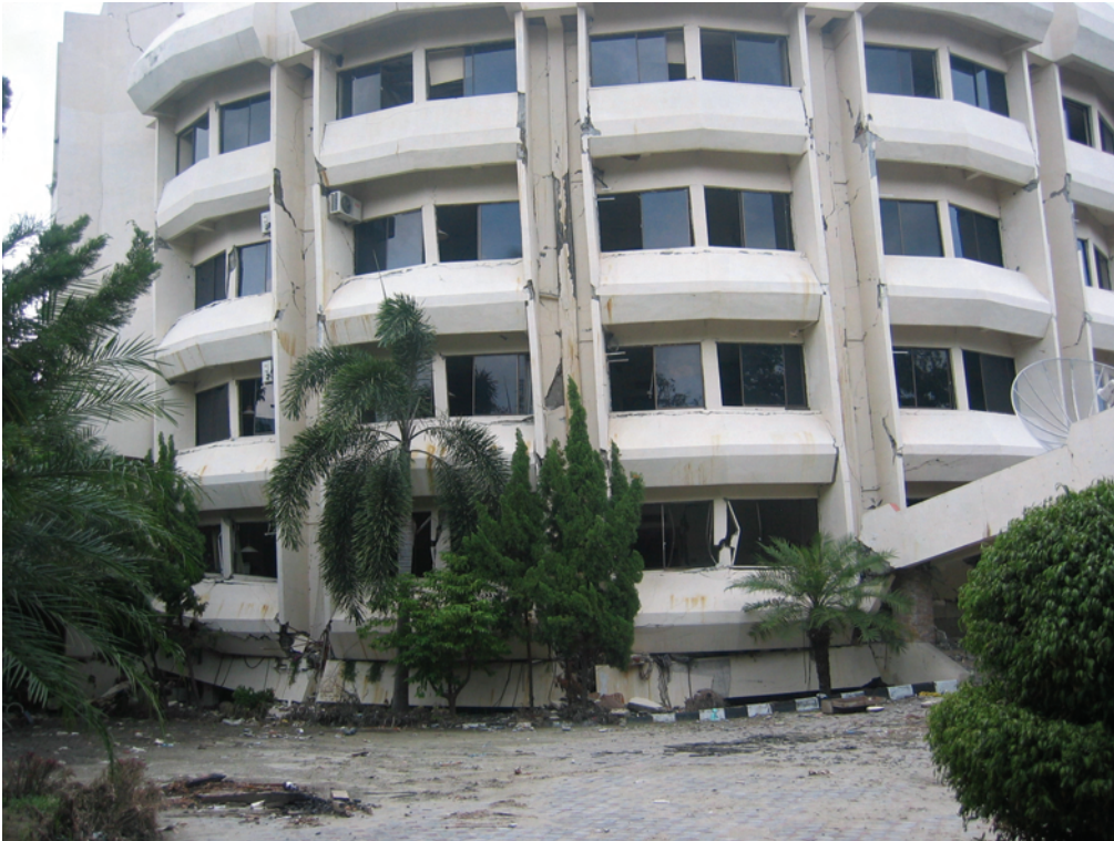
(b) Soft story failure
