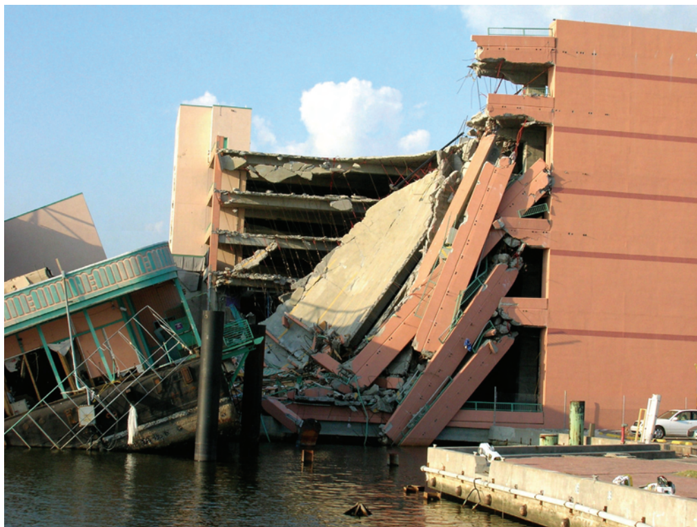
Figure 2-25 Progressive collapse of upper floors of a parking garage due to damage in lower level columns from impact of an adjacent barge-mounted casino (Hurricane Katrina, 2005).
