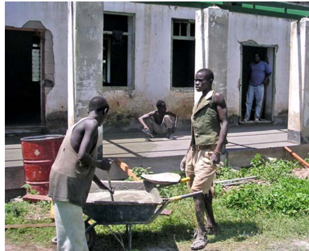
The Gbutala Secondary School in Maridi was rehabilitated with support from USAID. Photo: CARE
