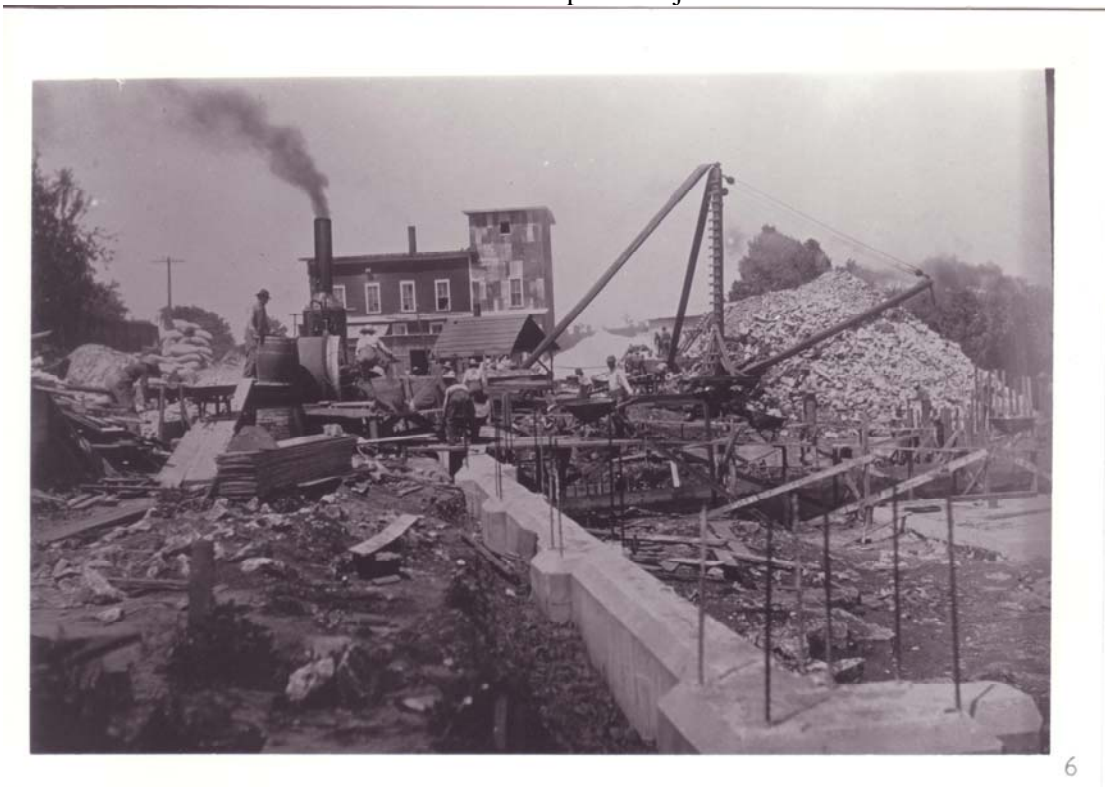
6/21/1910 – Concreting walls in basement of engine room. View from southwest corner of boiler room.
