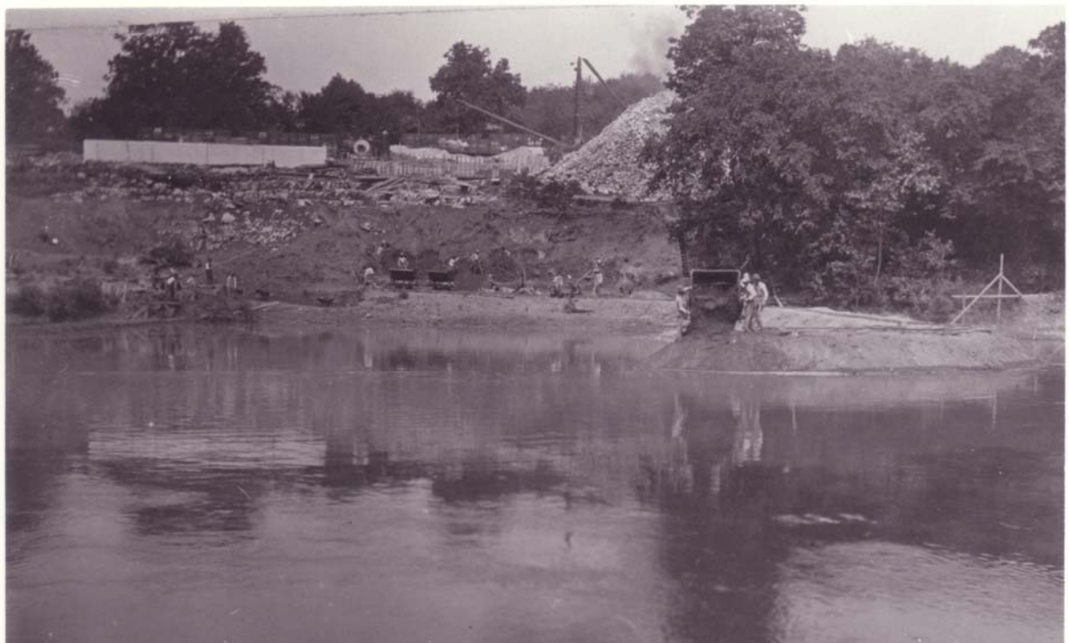
6/14/1910 – View from east bank showing method of building coffer dam from earth excavation from wheel pits.
