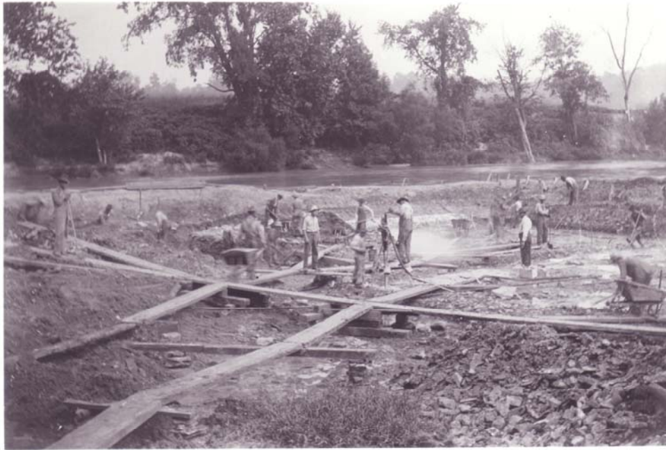
6/30/1910 – View of coffer dam from south end of wheel pits. Drilling rock at elevation 458. Coffer dam practically done.
