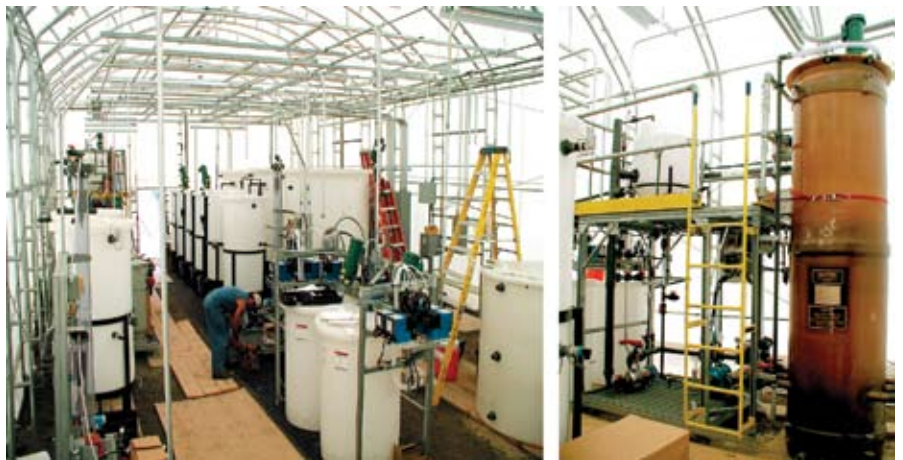
Near-source groundwater processing equipment for the biostimulation project.
