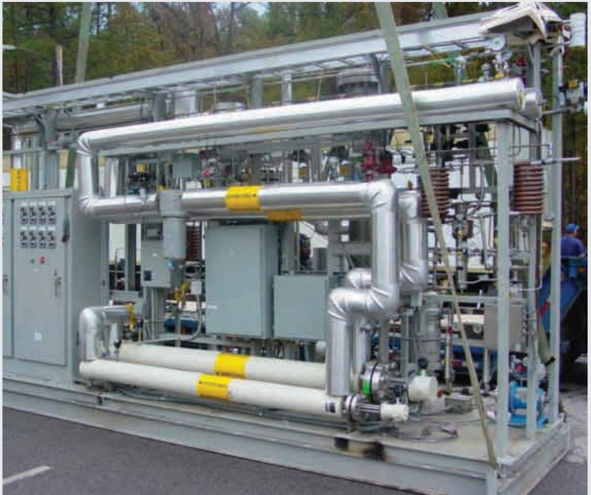
This direct sulfur recovery system test skid was integrated with a high-temperature desulfurization process unit (not shown) to convert recovered sulfur into a pure product for beneficial use.
