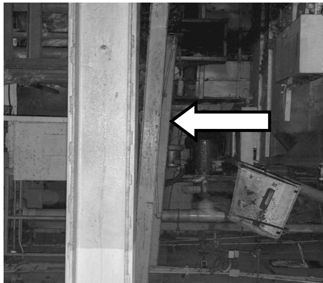
Figure 8. Bent support column in line 401 blend room.
