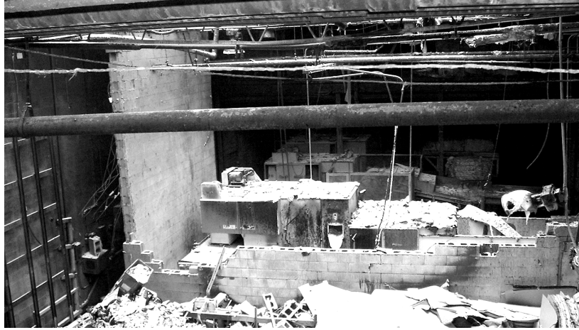
Figure 7. Collapsed firewall between lines 403 and 405.
