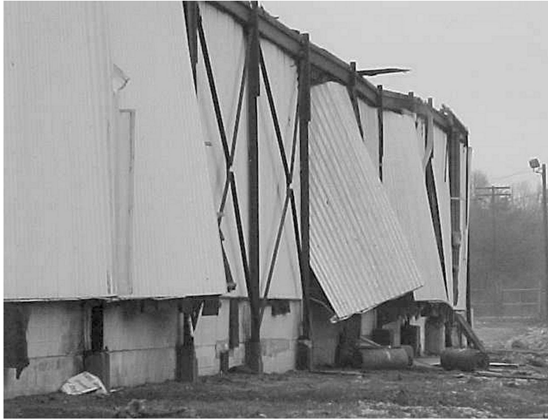
Figure 9. Explosion damage to exterior plant wall at southwest corner of building.
