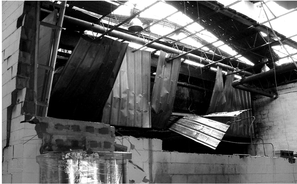
Figure 6. Collapsed firewall and metal panels at south end of line 405 blend room.
