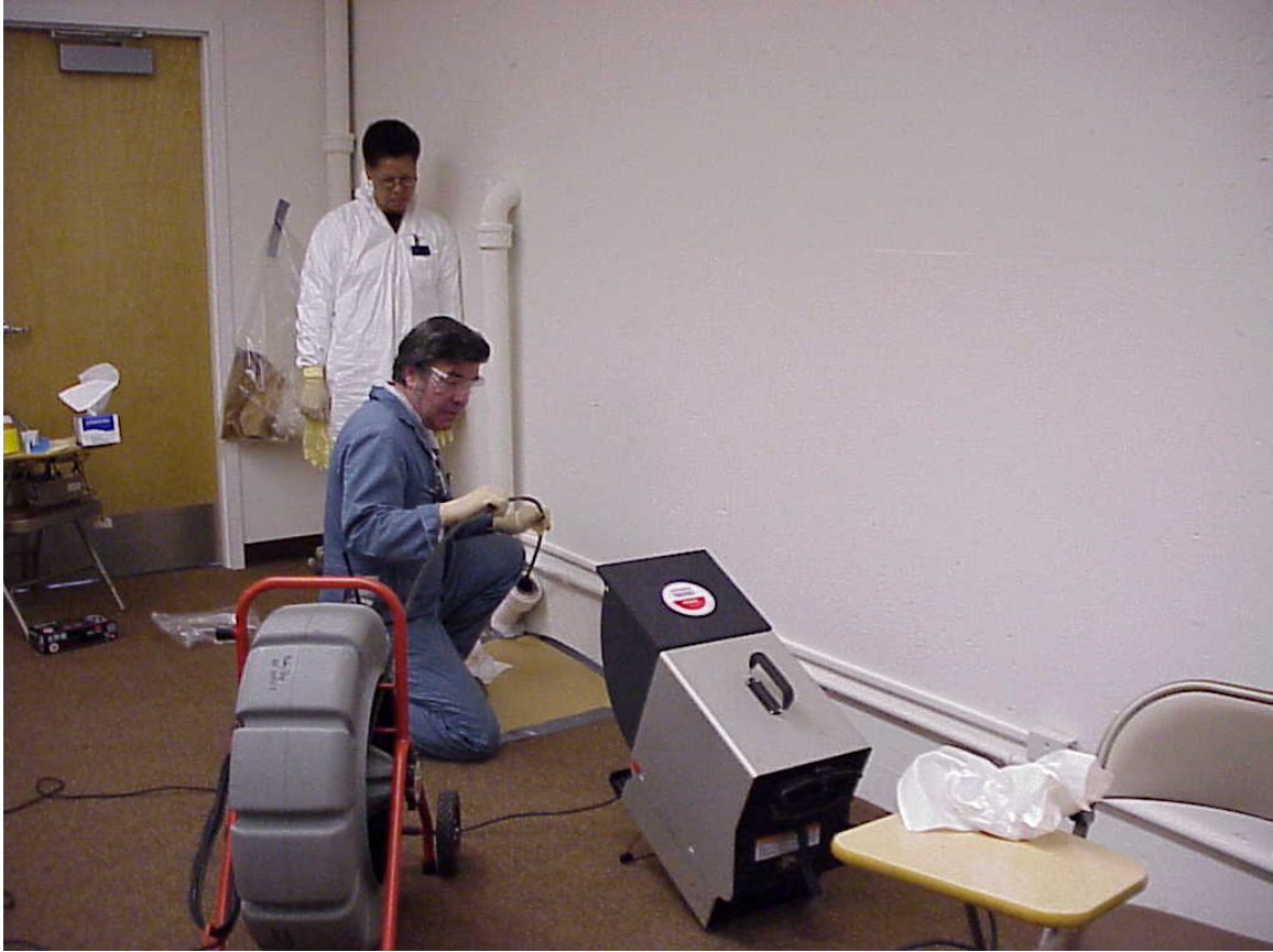
Figure 3. The condition of Building 4 sanitary sewer is being checked using a video camera.
