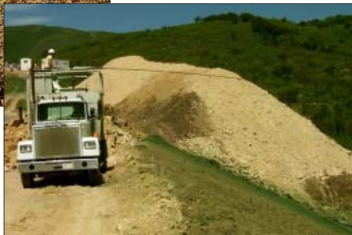
Large and accessible areas can be quickly covered with hydraulic seeding equipment.
