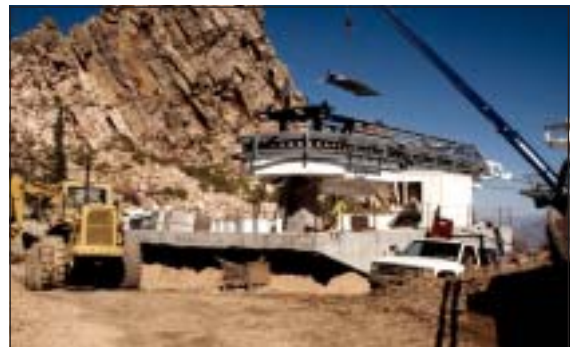
Excavations for ski lift terminal building foundations can yield large amounts of material that can be salvaged as fill for other activities.
