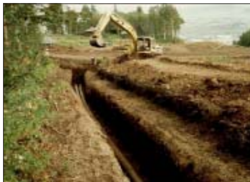
In trench excavation, subsoil should be placed above topsoil windrows to protect them from erosion and compaction.
