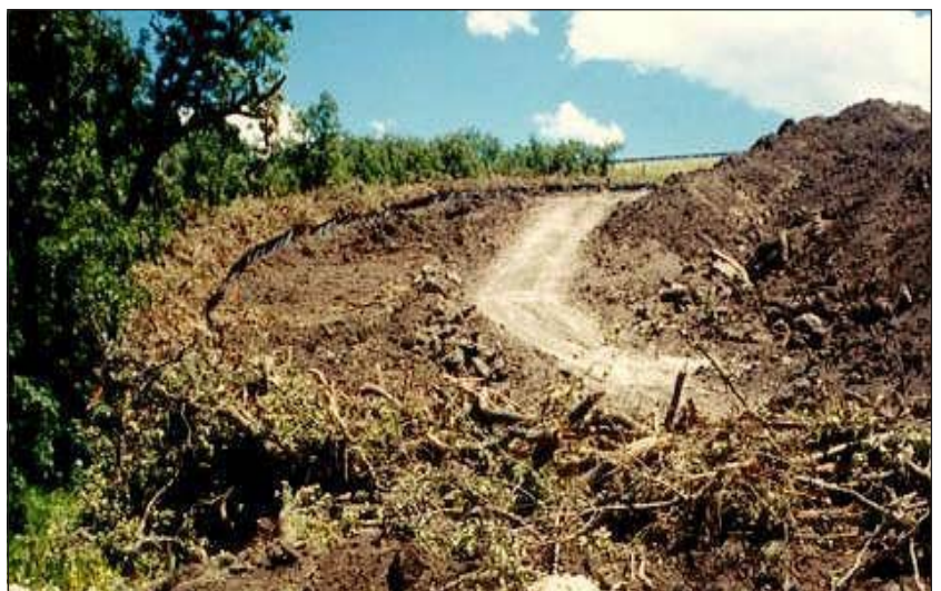
Where space is limited, less effective practices such as berms, silt fences, and slash barriers can be used together to replace a vegetation buffer strip.
