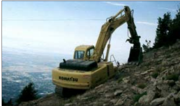
Full bench cut and end haul construction of a narrow low standard access trail.
