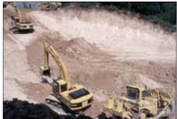
Ski lift terminal sites must be accessible by cranes and other large equipment.
