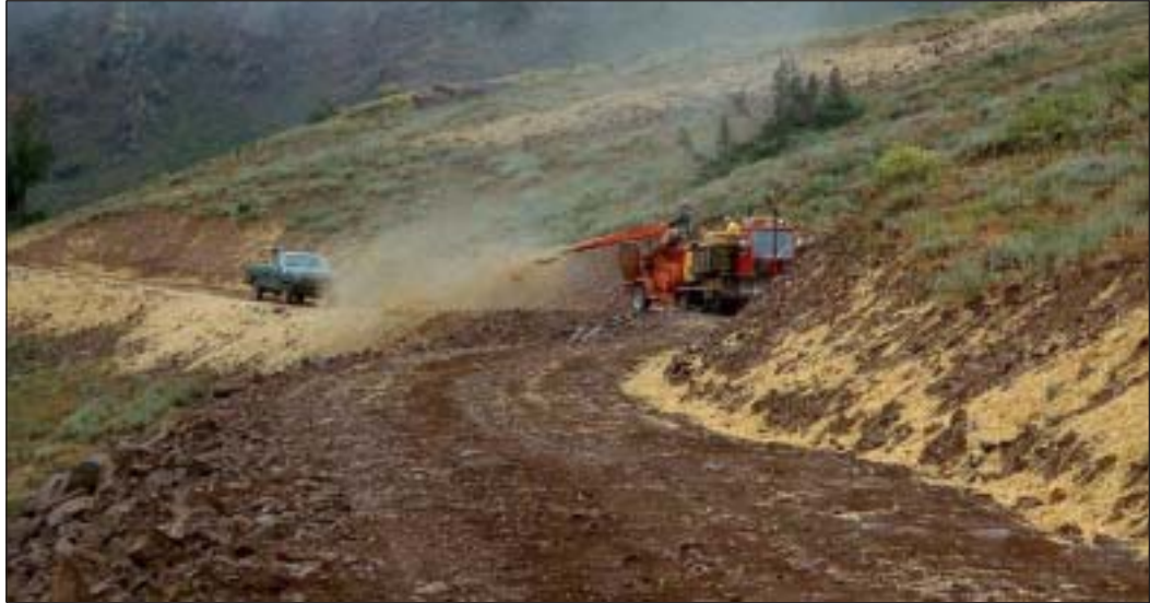
Road cut and fill slopes can be quickly covered with mechanical mulching equipment.
