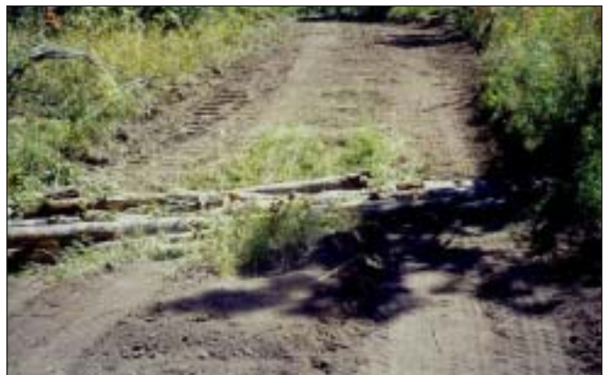
Logs can be used instead of culverts and fill to provide a temporary stream crossing for heavy equipment access across intermittent and ephemeral channels.
