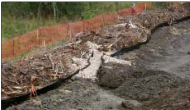
Silt fencing is usually placed on the level and parallel to the contour. Where a fence is sloping, relief outlets must be supplied at regular intervals.
