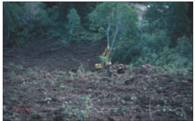
Vegetation clearing by trackhoe excavator leaving root mass and coarse debris ground cover.
