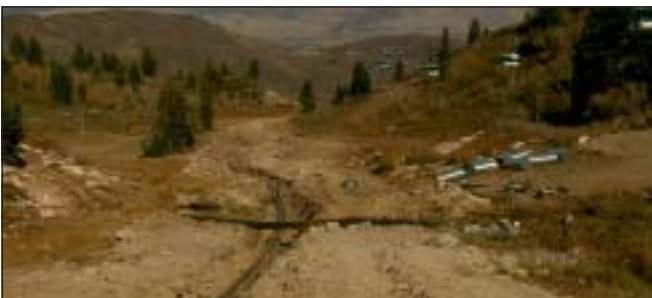
Temporary stream crossing culverts may need to be in place for several weeks until work can be completed and trenches backfilled.
