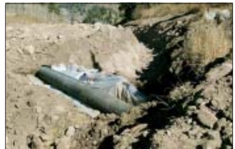
Several culvert sections can be joined where longer temporary stream crossings are required. Be sure to use plastic sheet lining to keep water leaks out of the trench.
