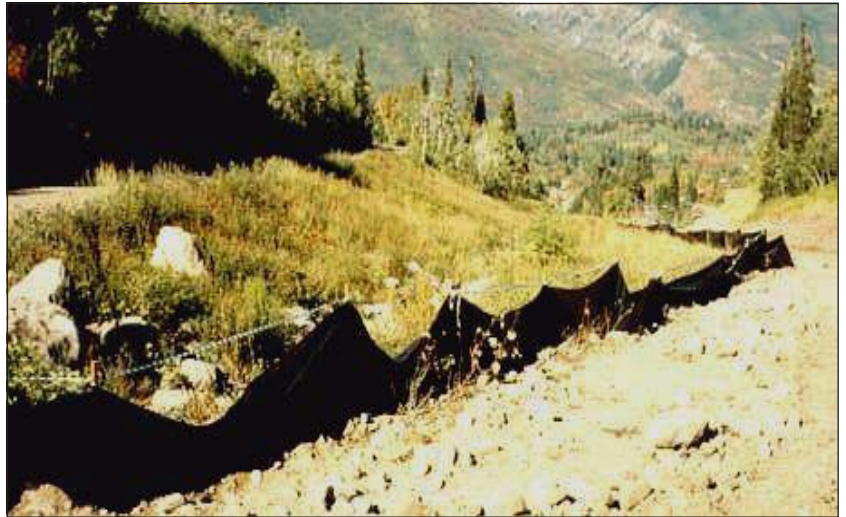
Vegetation buffer strips should vary in width based upon side-slope gradient. Where only a narrow strip is present, it should be supplemented with other sediment control practices such as silt fences or straw bale dikes.
