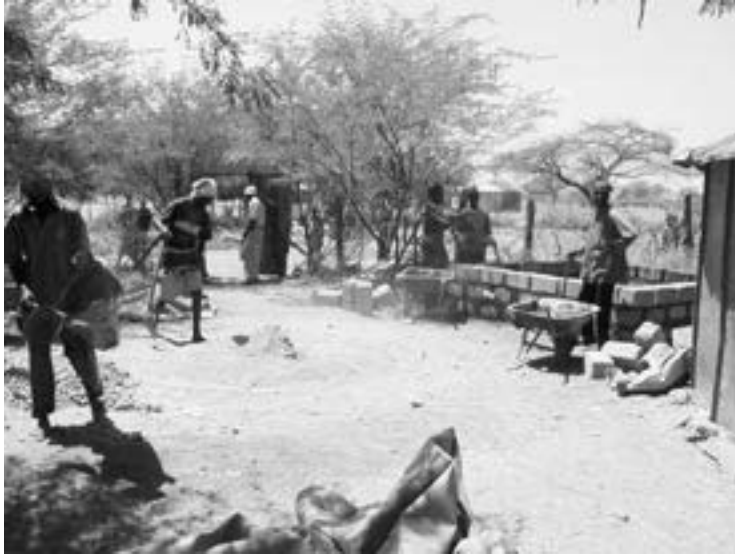
New construction or rebuilding of water and sanitation infrastructure, like this USAID/OFDA-funded project in northeast Kenya, helped the country transition to a recovery phase in FY 2002 (photo by Jack Myer, USAID/OFDA).
