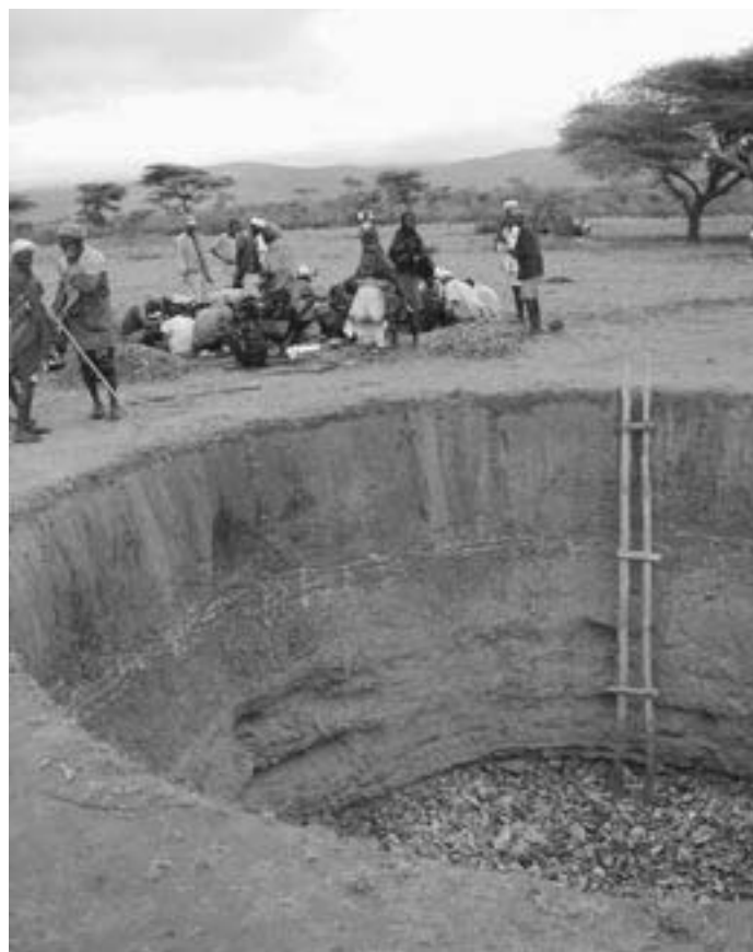
Residents in Yabello, Ethiopia look over the construction of a water cistern as part of a USAID/OFDA effort to decrease drought vulnerability in the region (photo by Bradford Adams, USAID/OFDA).
