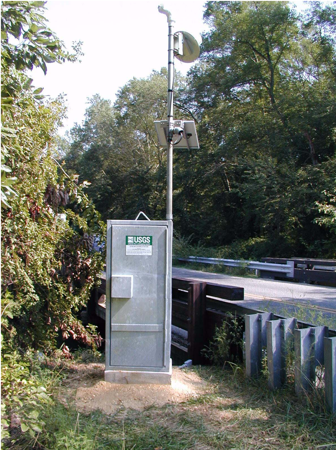
Figure 21. U.S. Geological Survey gage continuously monitoring the stage of the Cohansey River at Seeley, NJ. Photograph taken by Richard W. Edwards, 2003.
