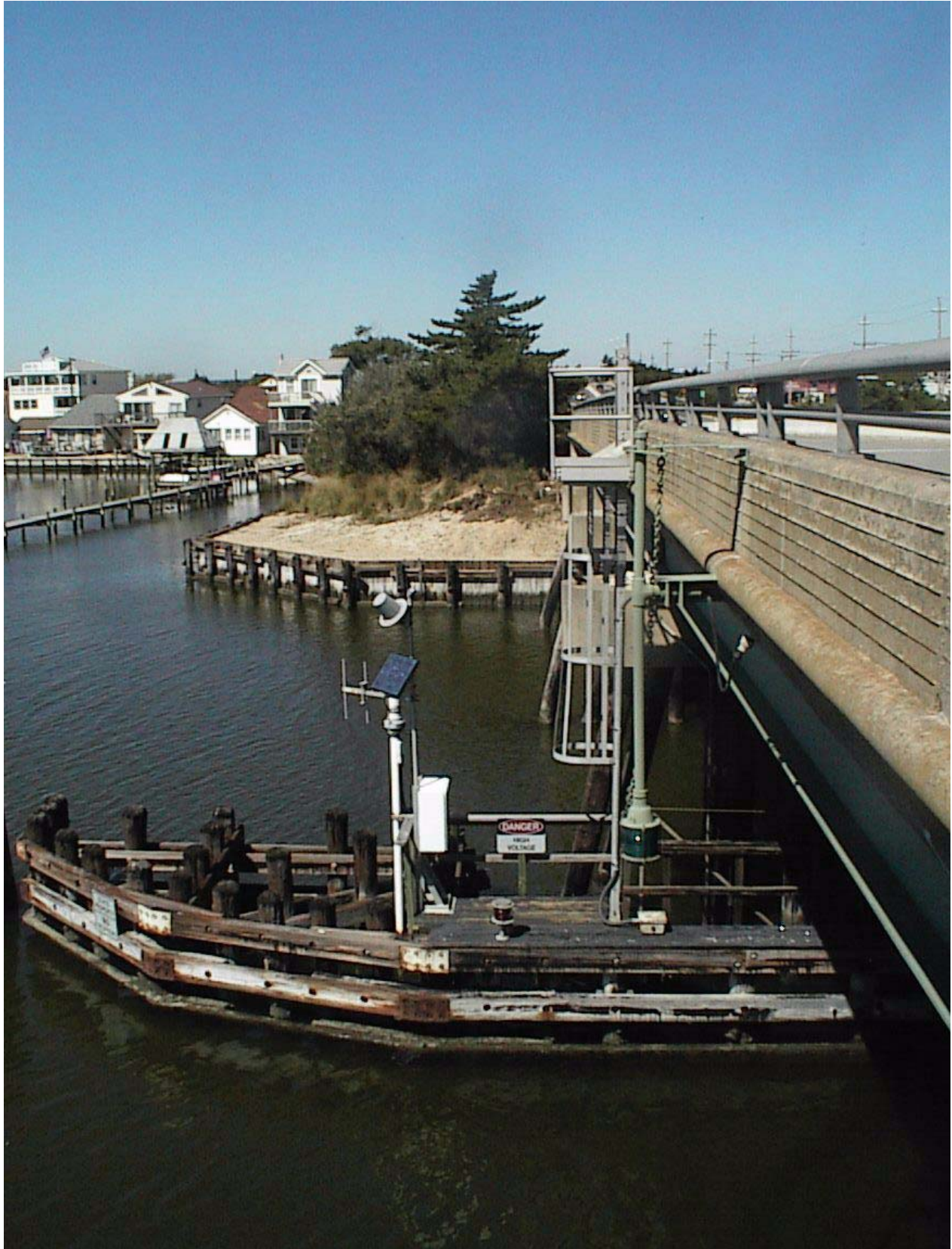
01409146 East Thorofare at Ship Bottom, NJ (file photograph, U.S. Geological Survey, West Trenton, New Jersey)
