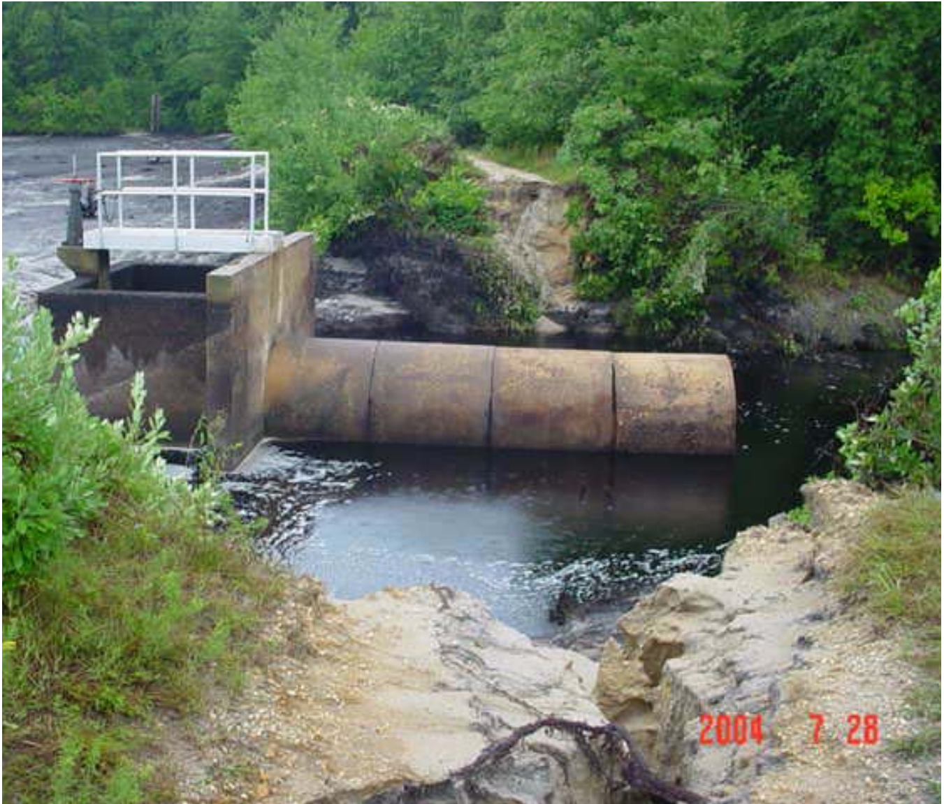
Aftermath of Lumberton Flood--Camp Inawendiwin Upper Dam washed out. adding to flooding along Friendship Creek in Tabernacle Township, during July 12-13, 2004 flood event. (file photograph, U.S. Geological Survey, West Trenton, New Jersey)
