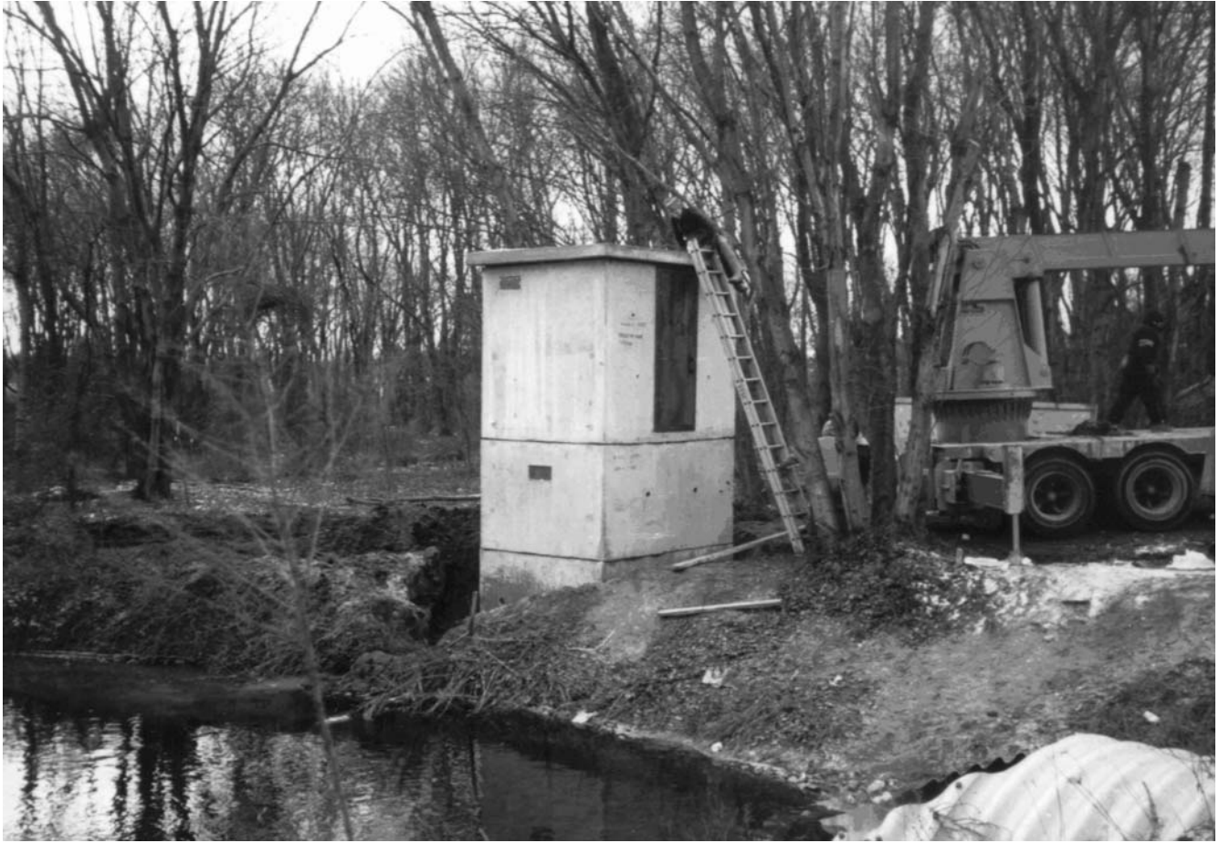
Figure 18. Construction of U.S. Geological Survey gage that will continuously monitor the stage of Little Ease Run near Clayton, NJ. Photograph taken by U.S. Geological Survey personnel, 1988.
