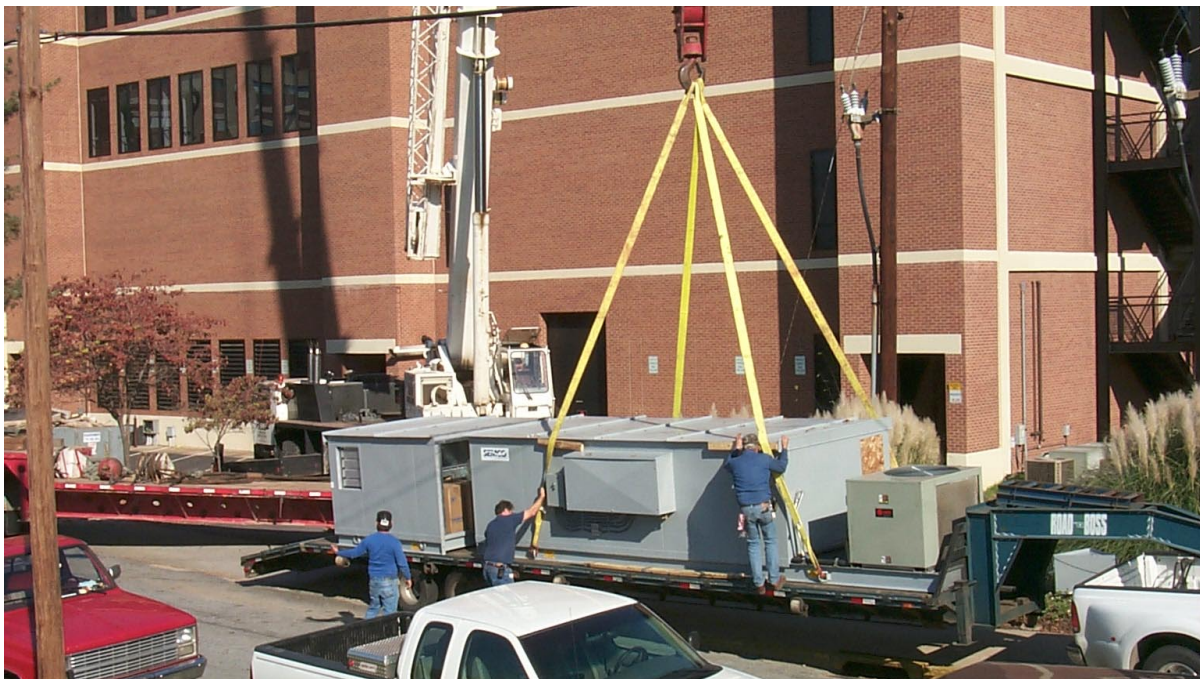
Fig. 17. The integrated SEMCO active desiccant system being installed at the Baker Building.
