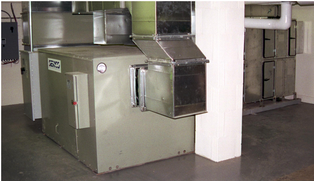
Fig. 5. The SEMCO FV total energy recovery module installation. Note active desiccant system with Climate Changer modules is shown to the right of the FV unit.
