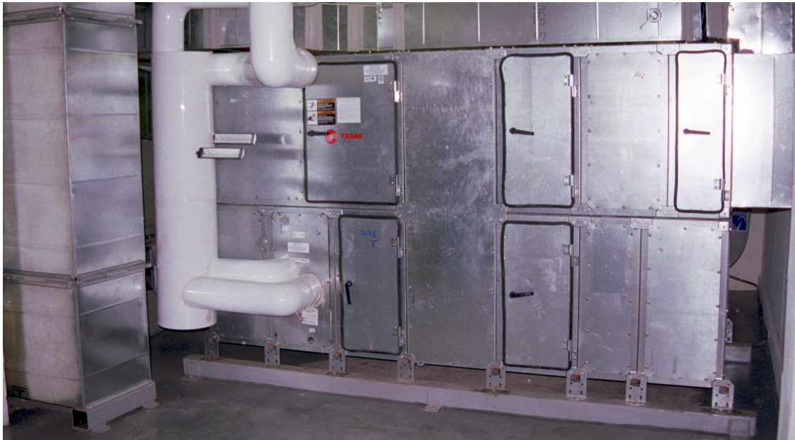
Fig. 7. Active desiccant system in the basement of Mary Hall showing standard Climate Changer modules attached to the SEMCO active desiccant wheel cassette.
