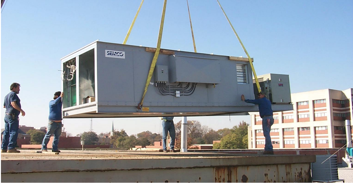
Fig. 18. The desiccant system rigged on existing pad. Gas piping/control panel shown.
