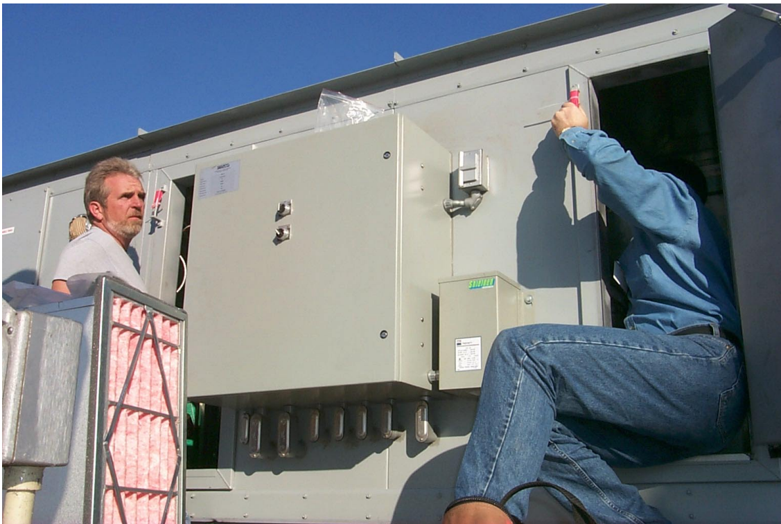
Fig. 19. The full electrical package, including the DDCs and communication software, factory-mounted as part of the integrated system. Note that high-efficiency filters were provided with the system to enhance the quality of the lab environment.
