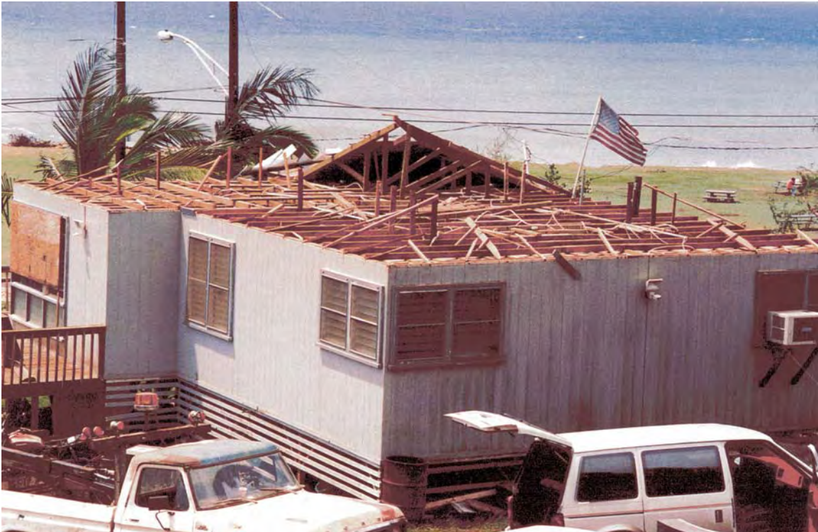
Hurricane Iniki roof damage to an unprotected home
