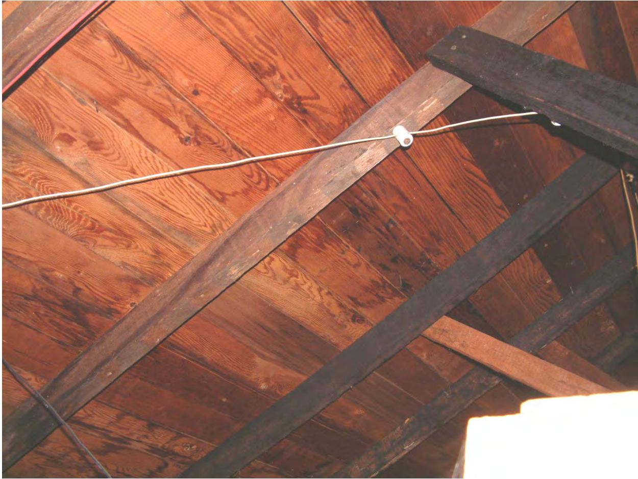
Figure 7: Example of an Older Roof Framed With Wood Trusses and Continuous Lumber Roof Decking (Viewed From Inside the Attic)
