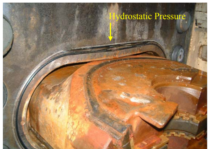
Failed bonnet seal caused by hydrostatic pressure forcing seal out of position.
