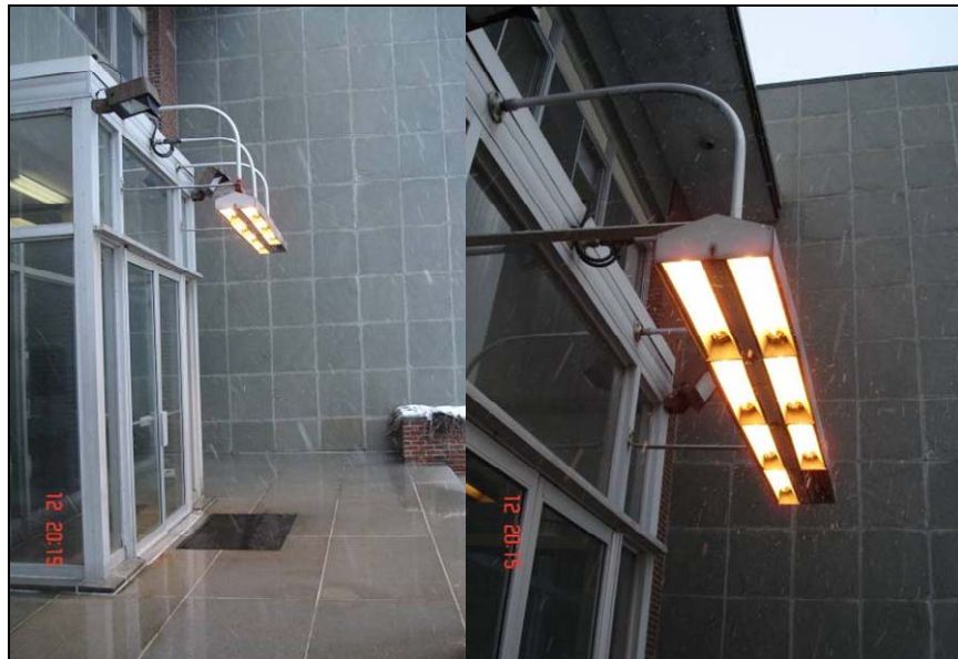
Figure 39. Infrared heaters above CRREL entrance.
