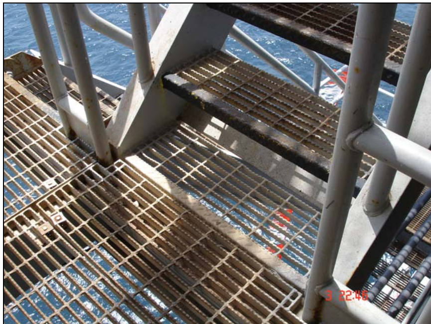
Figure 8. Open mesh walkways will accumulate ice and fill because of high collection efficiency.
