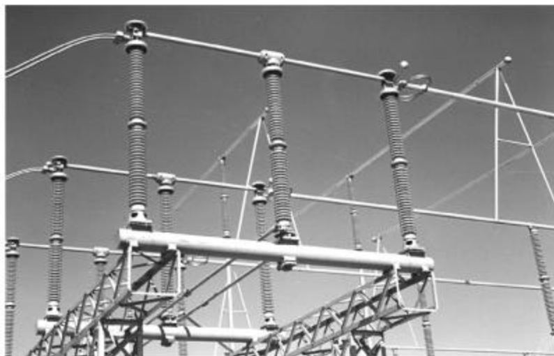
Figure 5-23: Horizontally Mounted Double-Break Switch. Note arcing horns and corona shields at blade contact points. Courtesy of Tuley & Associates, Inc.
