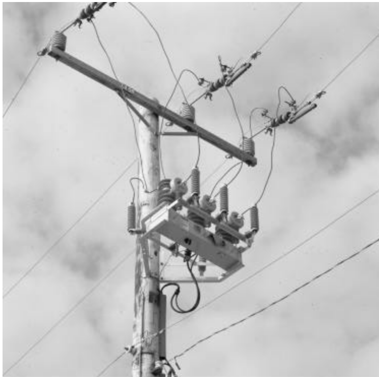
Figure 5-52: Mounted Recloser. Courtesy of Cooper Power Systems.
