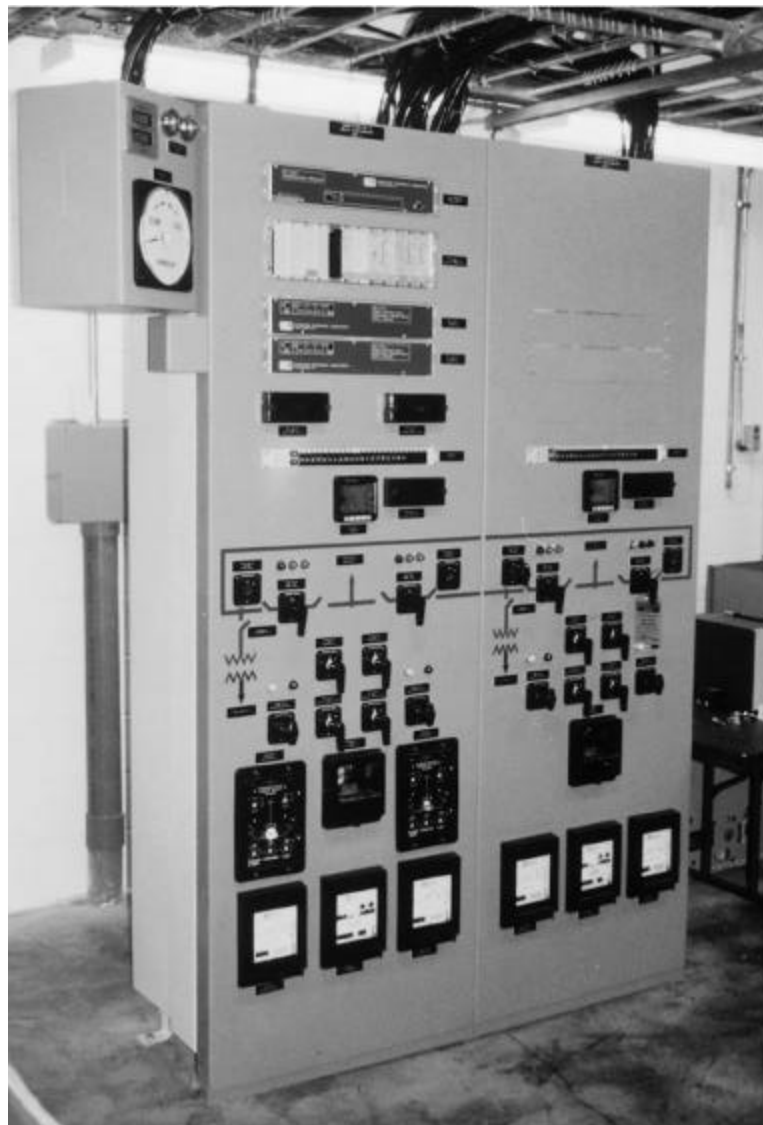
Figure 16-4: Typical Relay/Control Panel Layout. Note microprocessor, electromechanical relays, and mimic bus.
