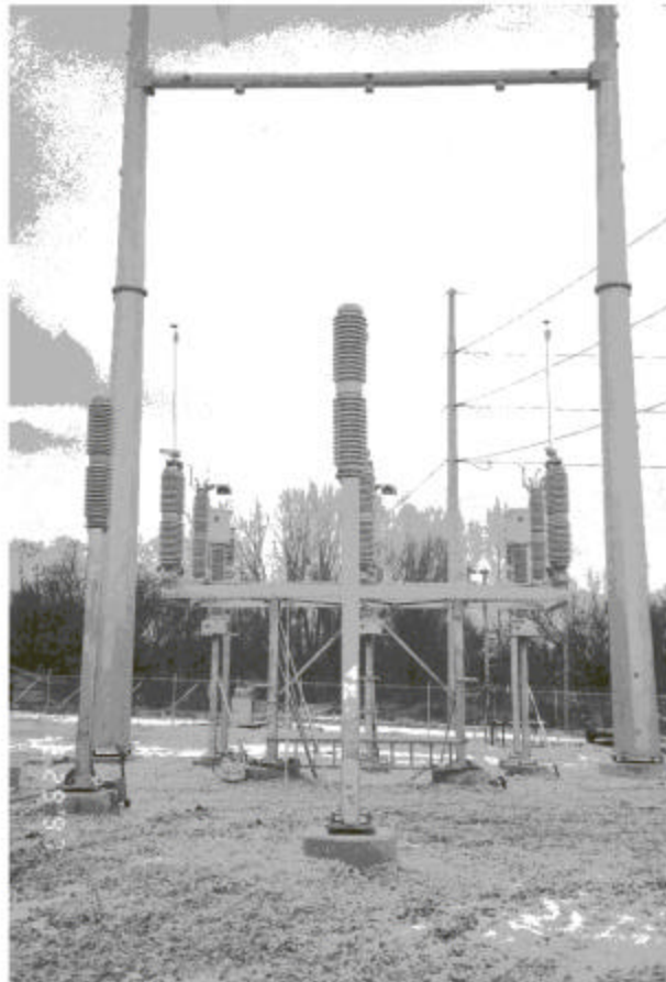
Figure 4-19: Station Post Insulator. Courtesy of Lapp Insulator Co.
