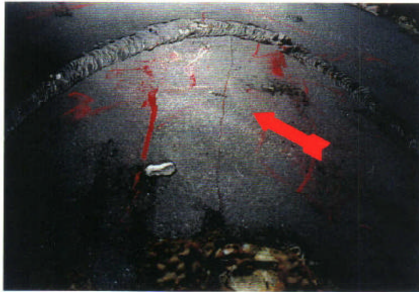
Figure 8.2: Crack that Results in a Flooded Member
