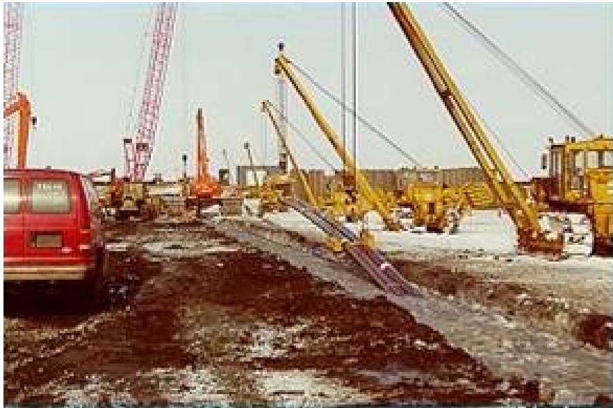
Figure 10-2: Gravel island approach excavation as sidebooms lower the Northstar pipeline bundle 50 ft to the seafloor (INTEC, 2000)
